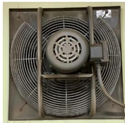
Garage Exhaust Fans
