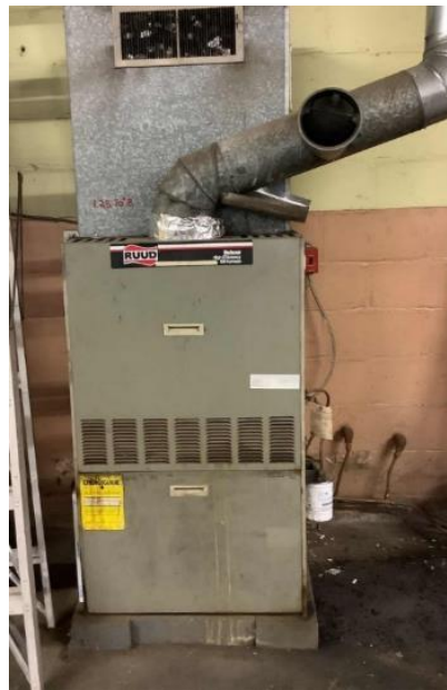
Central Supply Forced Hot Air Furnace
