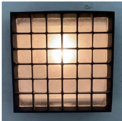
Toll Booth A19 Incandescent Lamp
