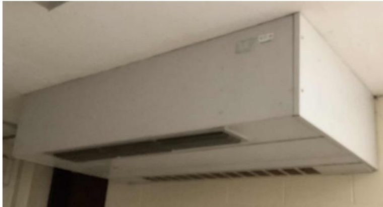
Liberty Grove Restrooms Electric Resistance Heater
