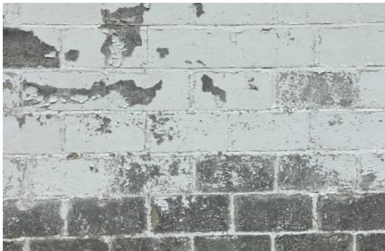
Central Supply CMU
