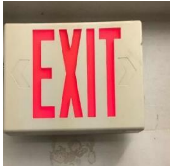
LED Exit Sign
