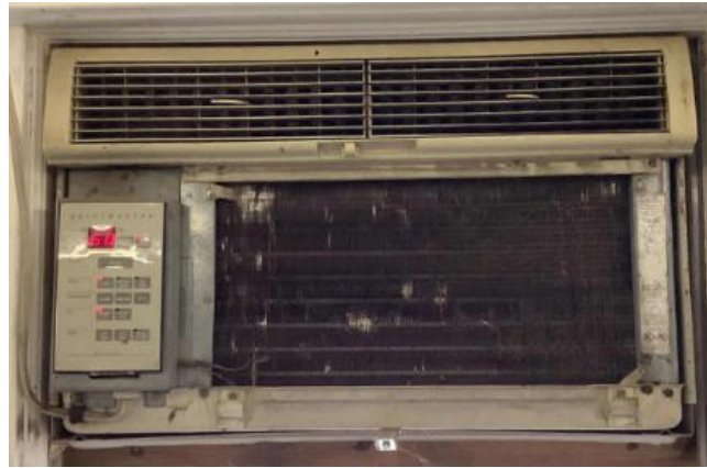
Central Supply 1.5-Ton Window AC Unit
