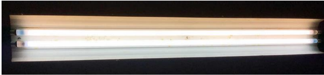
Potato Cellar 8-Foot Linear Fluorescent T12 Lamps
