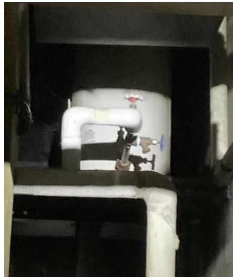
Liberty Grove DHW Tank
