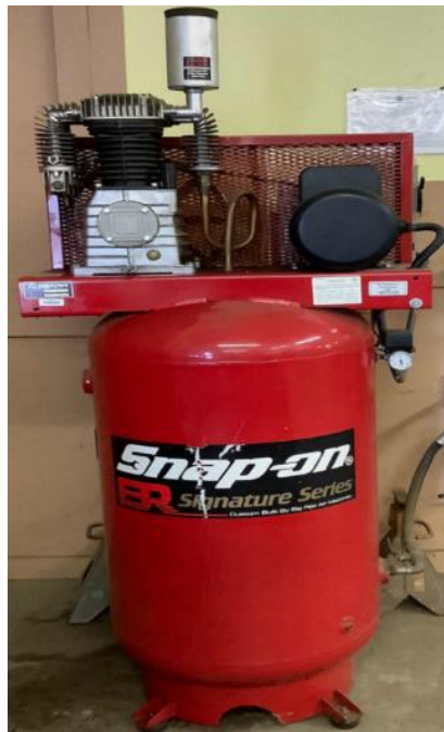
Central Supply Garage Air Compressor
