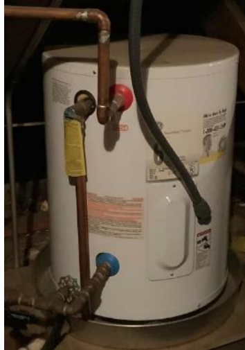
Central Supply DHW Tank
