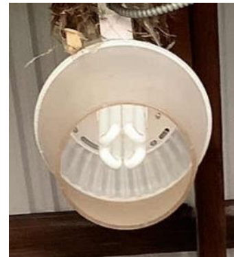
CFL Exterior Lights
