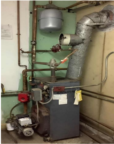
Central Supply Non-Condensing Hot Water Boiler
