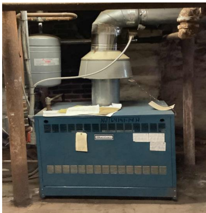
Propane Non-Condensing Boiler
