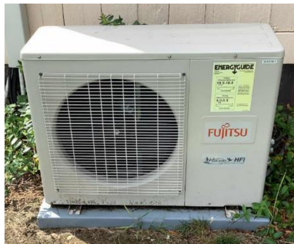
Packaged Air Source Heat Pump
