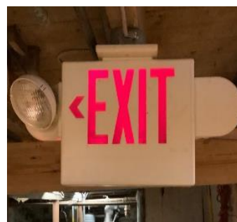
LED Emergency Exit Sign
