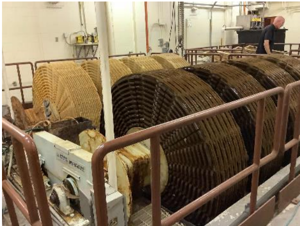
Rotating Biological Contactor
