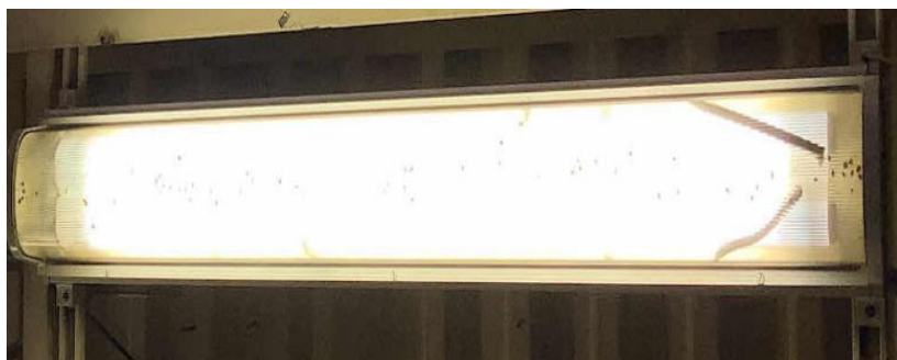
Storage Building 4-Foot Linear Fluorescent T12 Lamp
