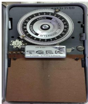
Exterior Lighting Time Clock
