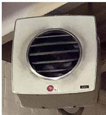
Storage Building Electric Resistance Heat
