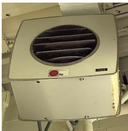
Sewer Plant Electric Resistance Heat
