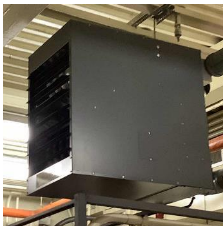
Sewer Plant Propane Fired Unit Heater
