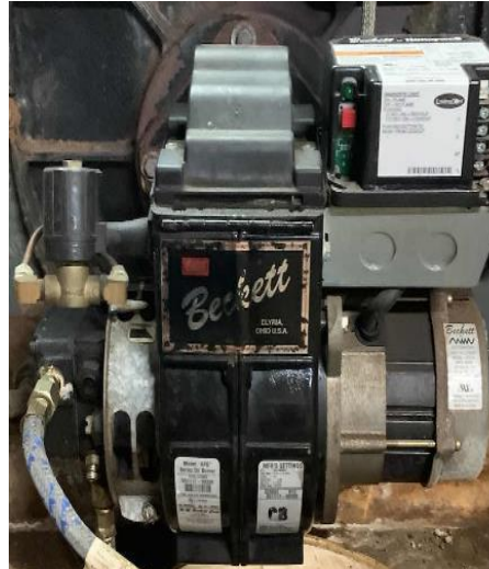
Tark House Beckett Oil Burner
