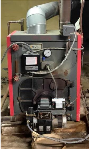
Tark House Steam Boiler
