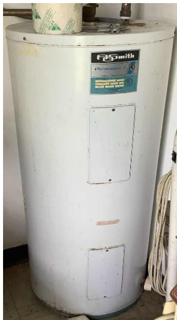
Craig House DHW Tank
