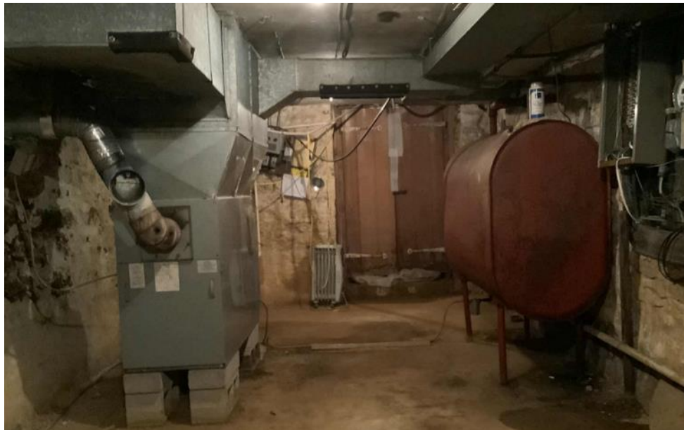
Craig House Forced Hot Air Furnace (Left) and No. 2 Fuel Oil Storage Tank (Right)
