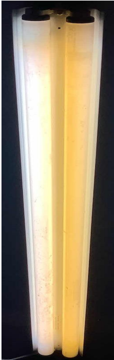
Tark House 4-Foot Linear Fluorescent T12 Lamps
