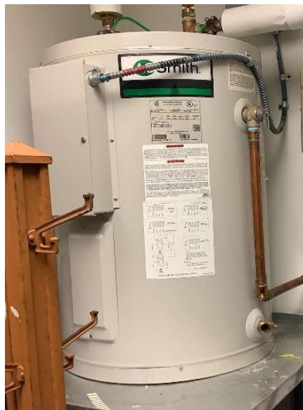
DHW Tank for New Visitor Center
