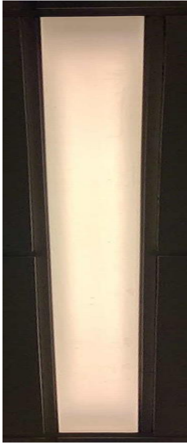
New Visitor Center 4-Foot Linear Fluorescent T5 Lamps
