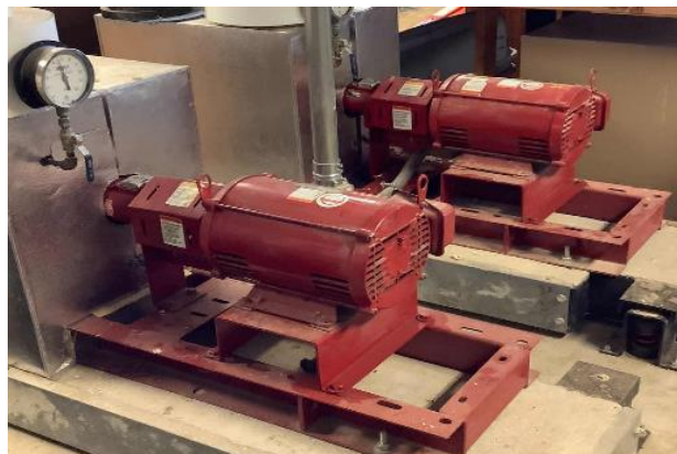
Ground Source Heat Pump Circulation Pumps
