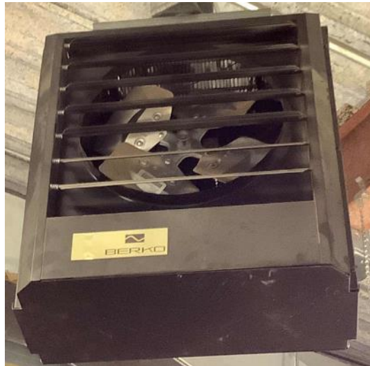
Server Room Electric Resistance Heating
