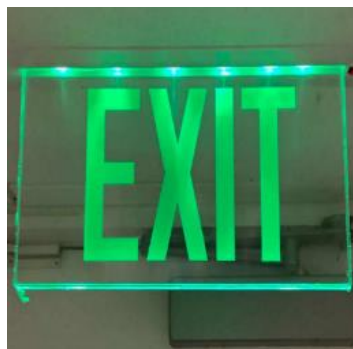
LED Exit Sign
