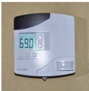
Occupancy based controls were installed in guest rooms.
