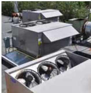
Intelligent controls regulate operation of rooftop air conditioning units.
