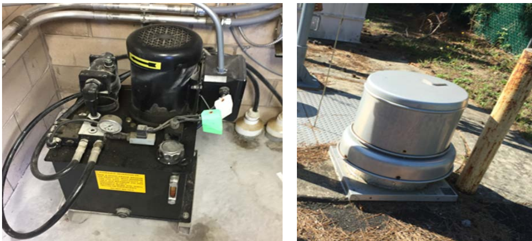
Image 4: Grinder Pump & Exhaust Fan
