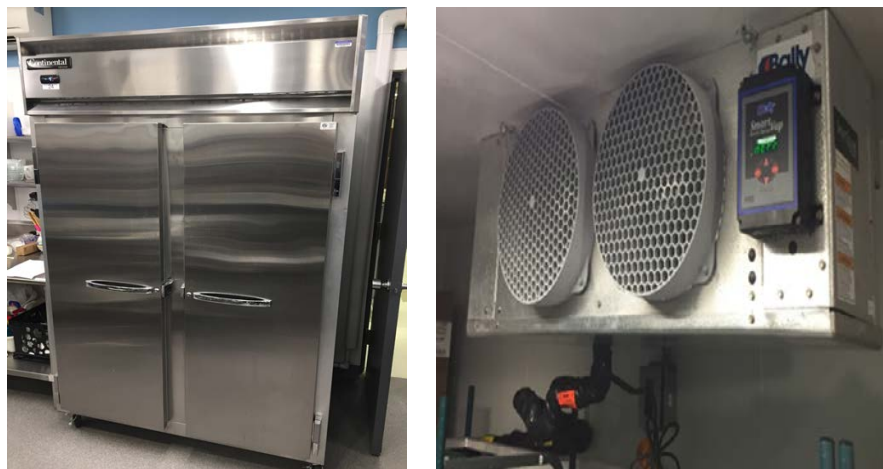
Standup & Walk in Refrigeration Systems
