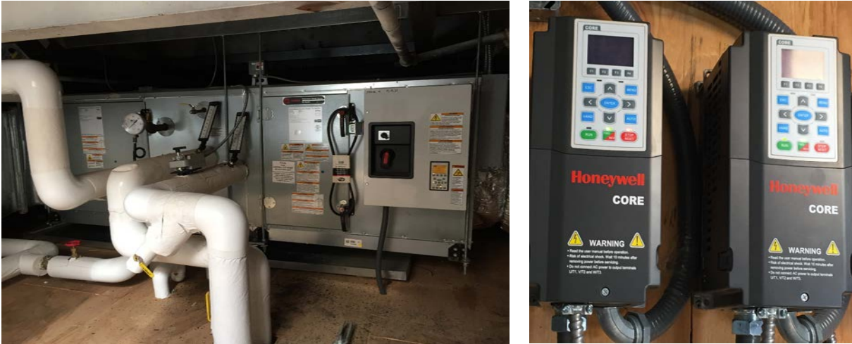
South Auditorium AHUs & VFDs
