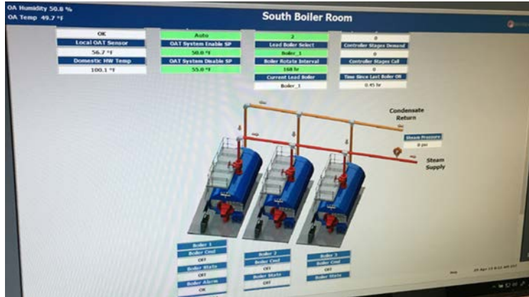
Steam Boilers EMS Control System
