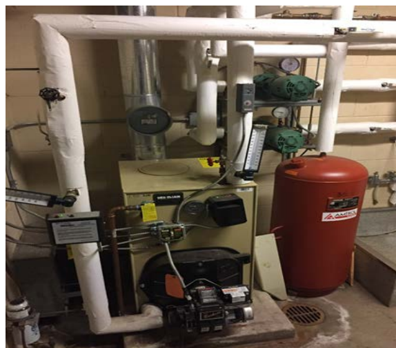
Oil Fired Boiler
