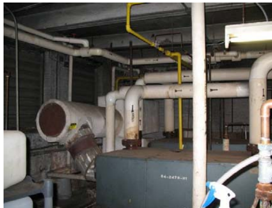
Old steam boilers in mechanical room
