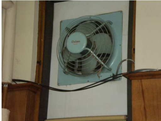
Plastic bag covering fan in downstairs classroom #16
