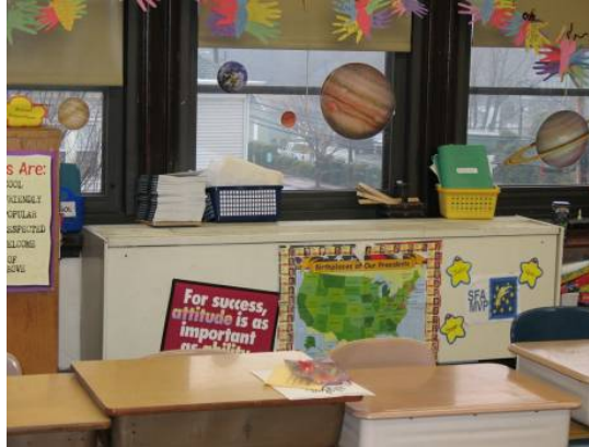
Single pane windows with plexiglass inserts
