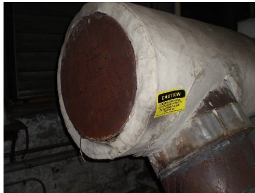
Caution notice of asbestos on boiler flue
