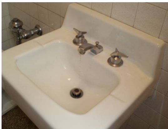
Lavatory faucet dripping in boy's restroom
