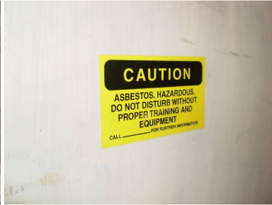
Asbestos Warning on Boiler
