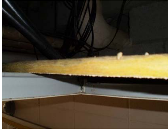
Duct board insulation approximately R2 – R3
