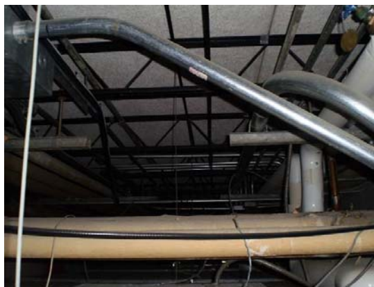
Plenum above ceiling
