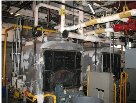
Boilers in Mechanical room
