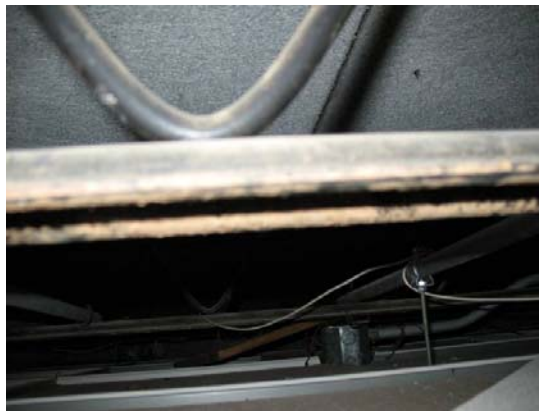
Plenum above ceiling
