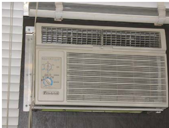
Window air conditioning unit
