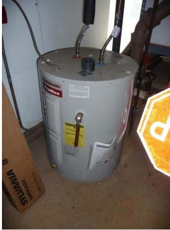
DHW electric heater
