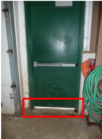
Light emitting through missing/worn weather stripping (typical at doors)
