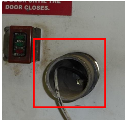
Oversized diameter hole with one wire running through none caulked and none insulated penetration (Typical improperly air-sealed penetration)
