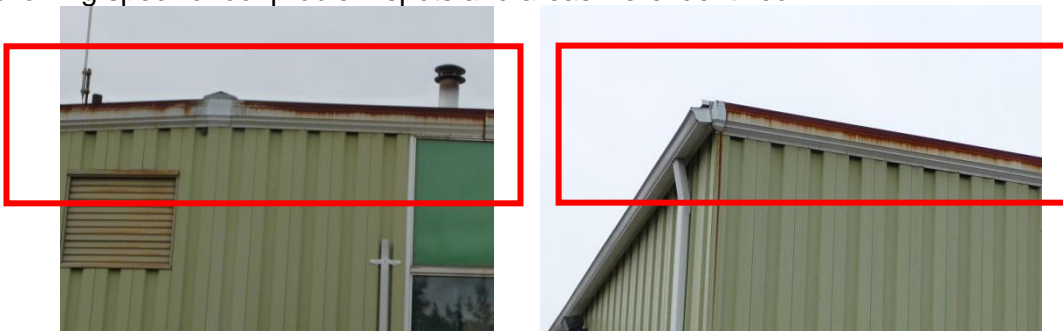
Garage roof has rust damage attributed to uncontrolled moisture leakage and due to the metal roofing material approaching the end of its useful lifespan.
