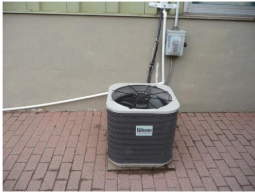
Break & Locker Rooms condenser
