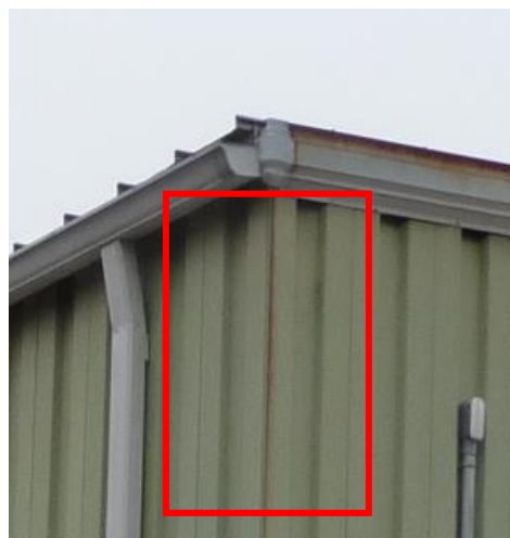
Corroded seams in wall due to rust
