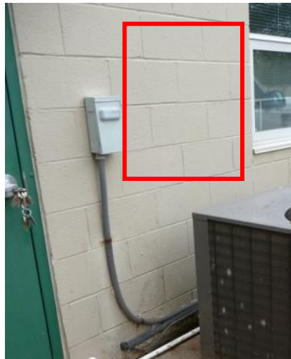
Exposed CMU blocks do not provide effective insulation in the office building
