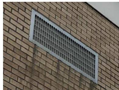
Outside Air Intake
