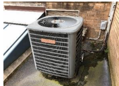
Heat Pump Condensing Unit
