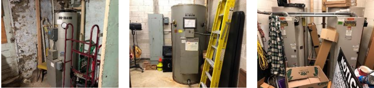
Electric Storage Water Heaters
