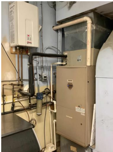
AHU in first floor Lounge
