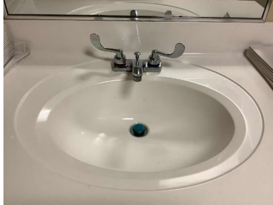
Typical Restroom Sink
