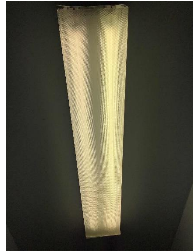
Linear Fluorescent T8 Lamps in a Surface mounted Fixture
