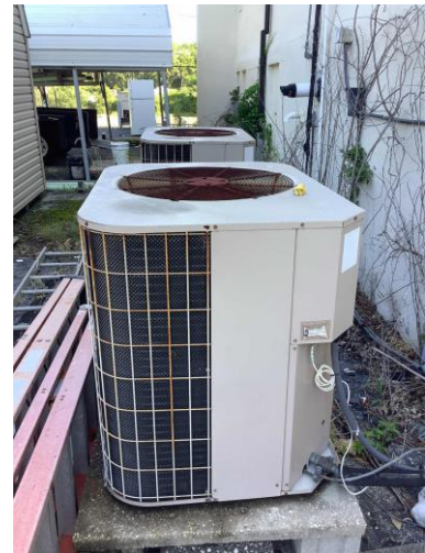
Outdoor Condensing Units
