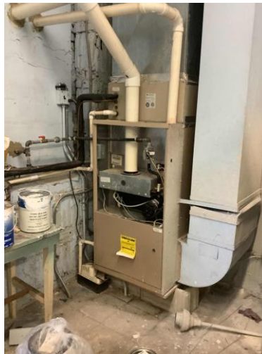
AHU in Paint shop
