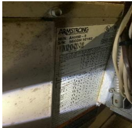
Air handling Unit Nameplate
