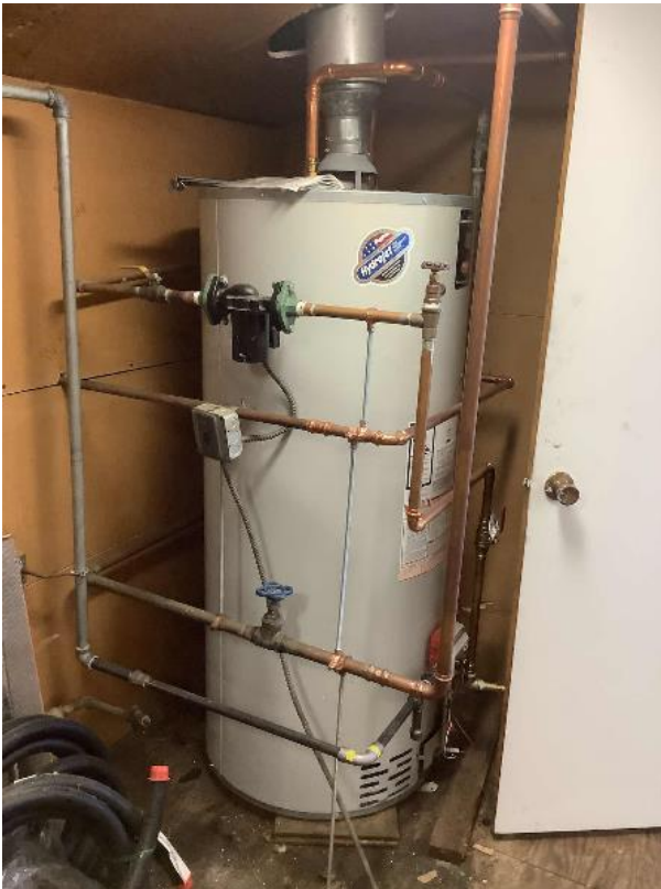
Domestic Hot Water Tank
