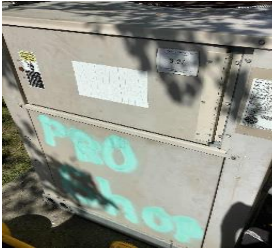
Pro Shop Outdoor Condensing Unit
