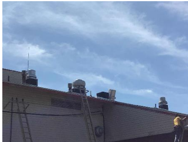
Rooftop Exhaust Fans
