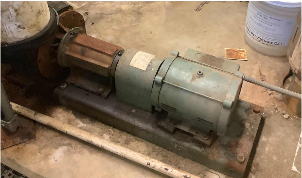
Chilled Water Pump - Annex
