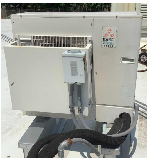
Mini-Split HVAC Unit
