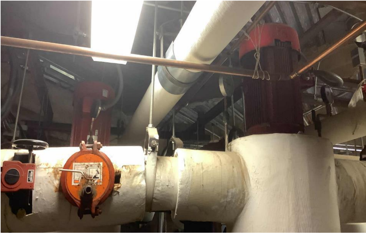
Chilled Water Pumps – Main Building
