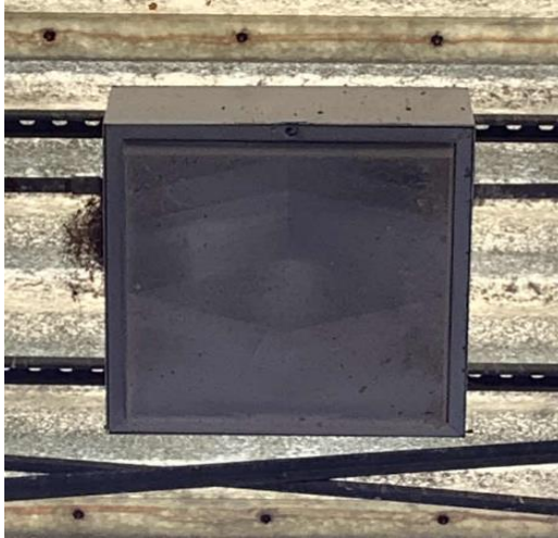
Exterior HPS Fixture
