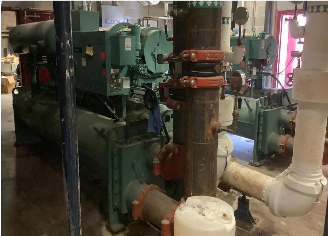
Water-cooled Chillers – Main Building
