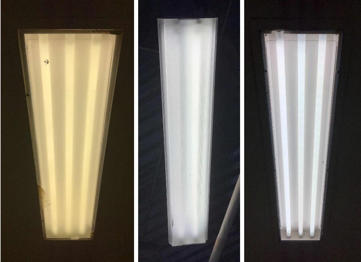
Fluorescent T8 Fixtures
