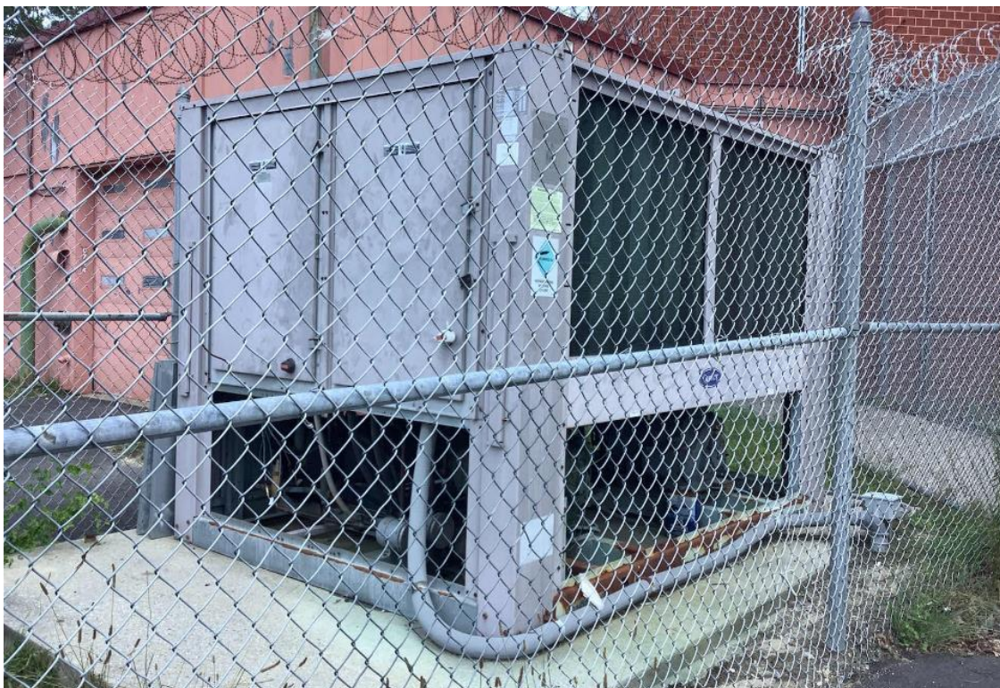
Air-cooled Chiller - Annex
