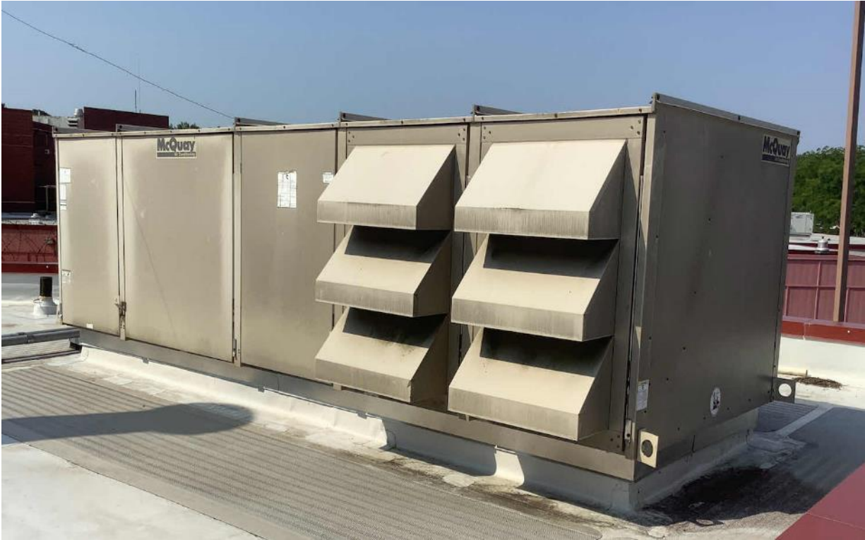
Packaged Unit - Annex
