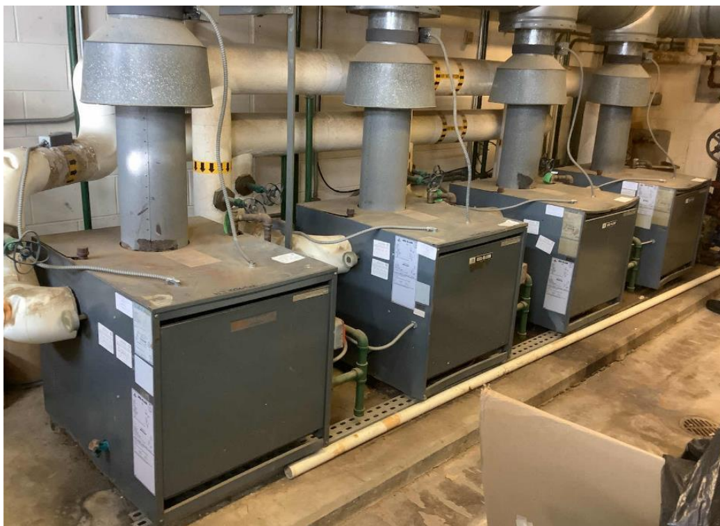
Hot Water Boilers – Annex
