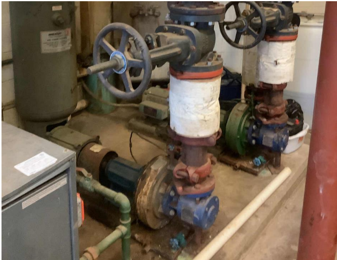
Heating Hot Water Pumps - Annex
