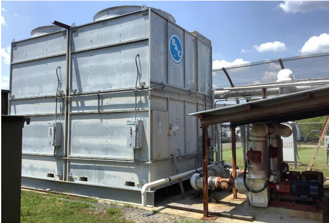
Cooling Towers and Condenser Water Pumps – Main Building
