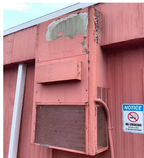
Through-the-Wall HVAC Units
