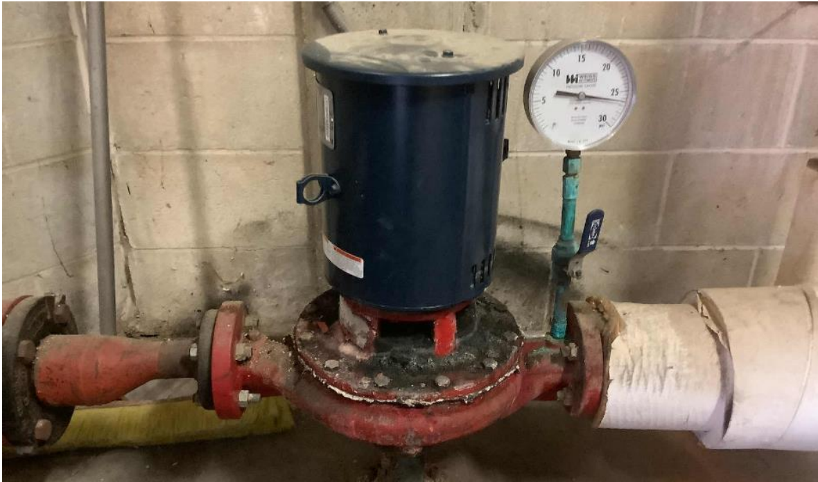
Heating Hot Water Pump – Main Building
