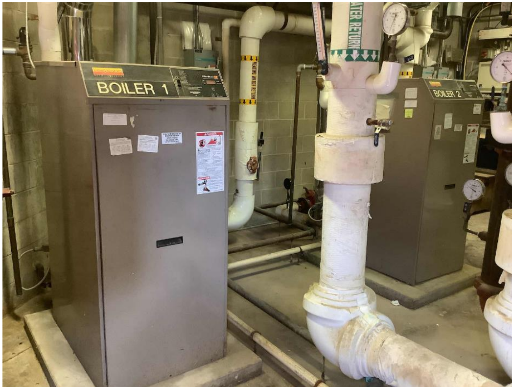
Hot Water Boilers – Main Building
