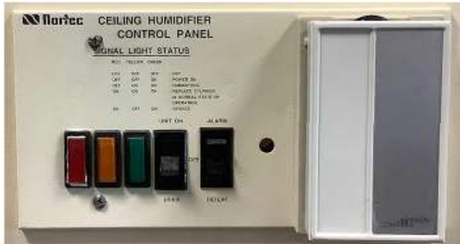
Humidifier Control Panel
