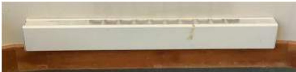
Electric Baseboard Heat
