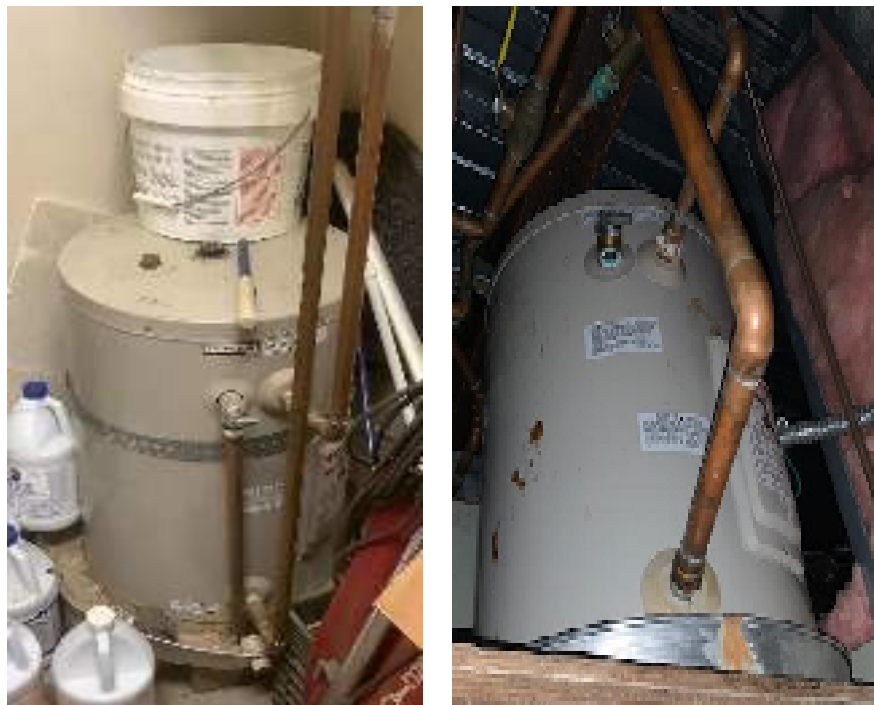
Roof Access & Above Ceiling DHW Tank
