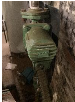
DHW Circulation Pump
