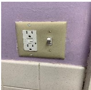
Bathroom Wall Switch
