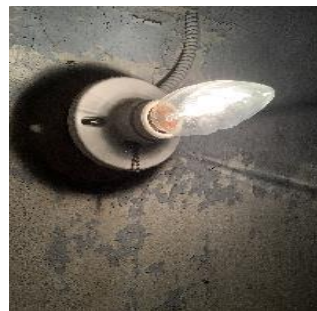
Halogen Bulb with a draw String in Basement
