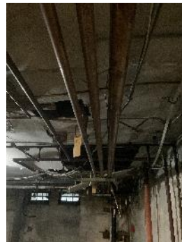
Uninsulated HHW Supply Piping
