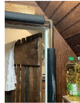
Apartment Kitchen Closet DHW pipes
