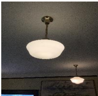
Pendant Fixture with A19 LEDs (Present in most of the classrooms)
