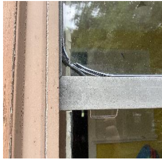
Storm Window Seals in poor condition
