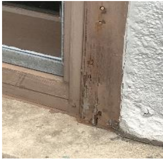
Wooden Window Frames in poor condition
