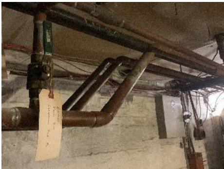
Uninsulated HHW Supply Piping
