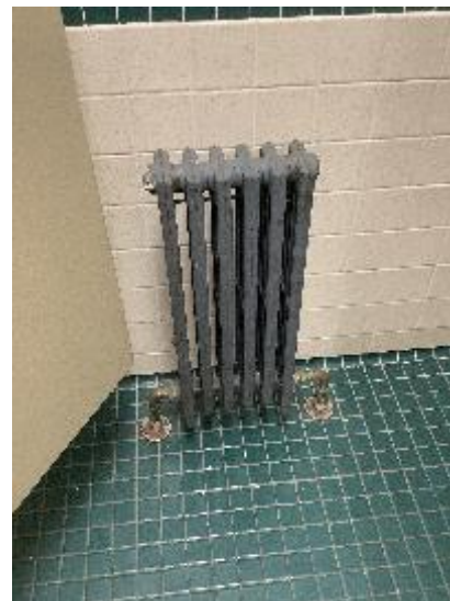
Cast Iron Radiator
