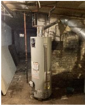
DHW Heater and uninsulated piping
