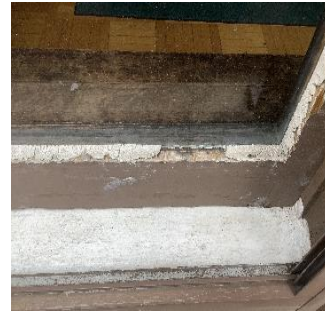
Window Seals in poor condition
