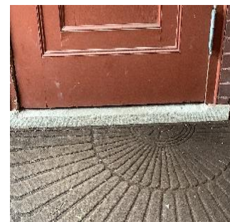
Gap under Front Door
