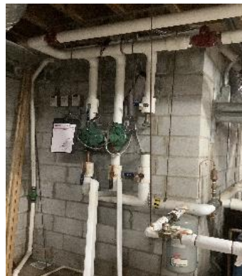
Two ¼ hp HHW Pumps
