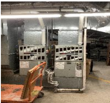
Furnaces 1A, 1B
