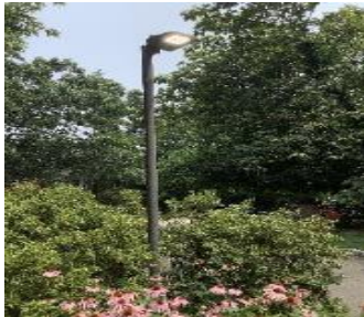
Parking Lot Pole Light
