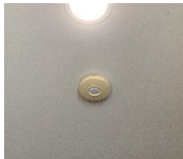
Hallway Ceiling Mounted Occupancy Sensor
