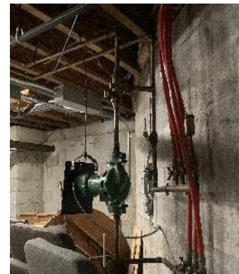
1/3 hp HHW Pump and Uninsulated Piping
