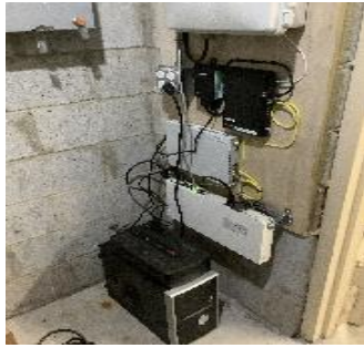
Basement Electrical Room
