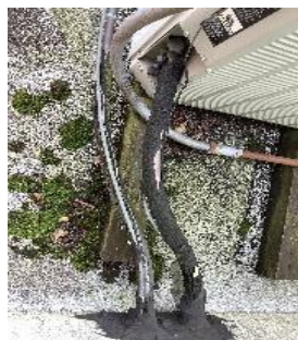
Moss on the Roof
