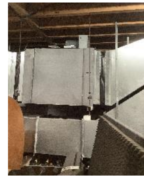
Furnaces 3A, 3B
