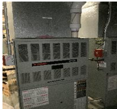
Furnaces 2A, 2B
