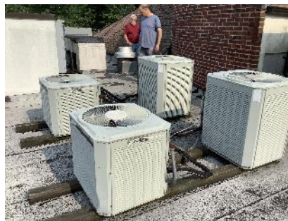
Condensing Units 1A, 1B, 2A, 2B
