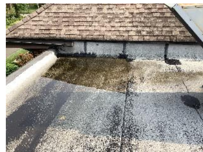
Standing Water on the Roof
