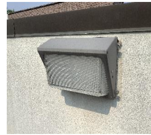
Roof LED Wall Pack
