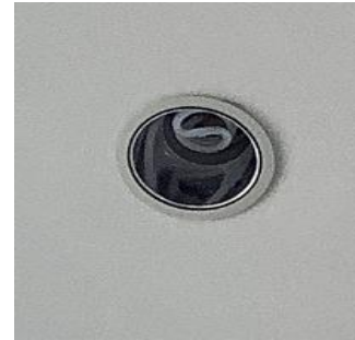
High Ceiling CFL in Recessed Can
