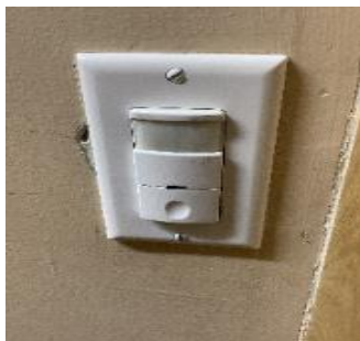
Wall Occupancy Sensor and Switch
