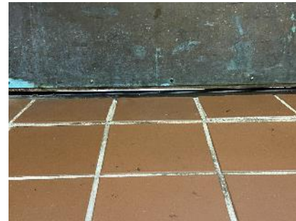
Kitchen Door Gap
