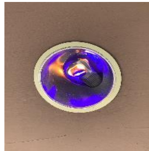
Damaged and Overheated 17-Watt LED
