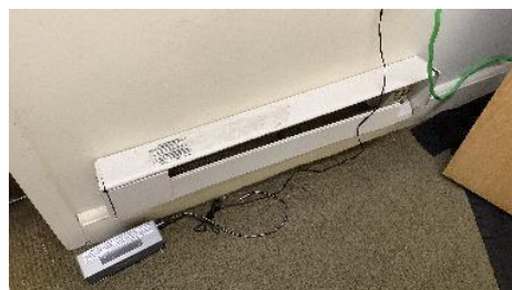
Stairwell Electric Radiator
