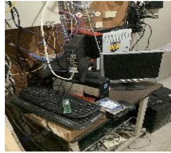
Basement Electrical Room
