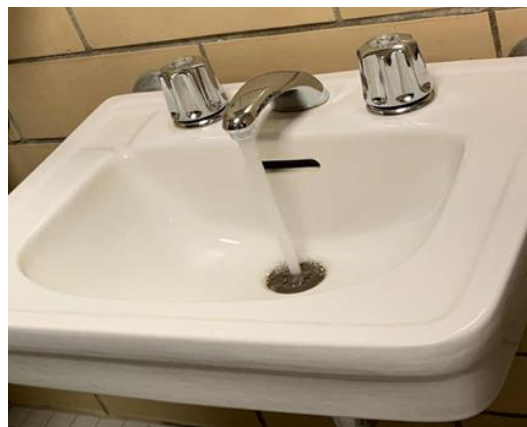
Typical Restroom Sink
