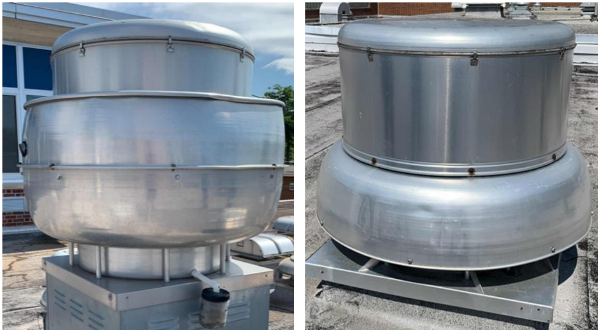
Kitchen Hood and Dishwasher room Exhaust Fans
