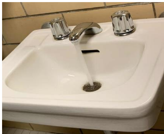
Typical Restroom Sink
