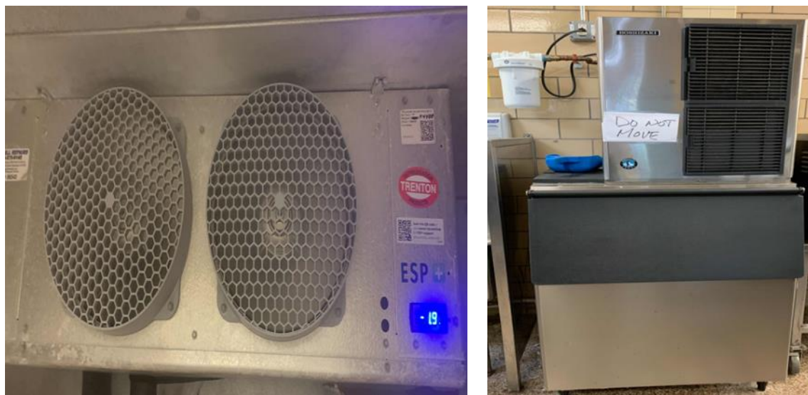
Evaporator (Walk-In Box) and Ice Machine
