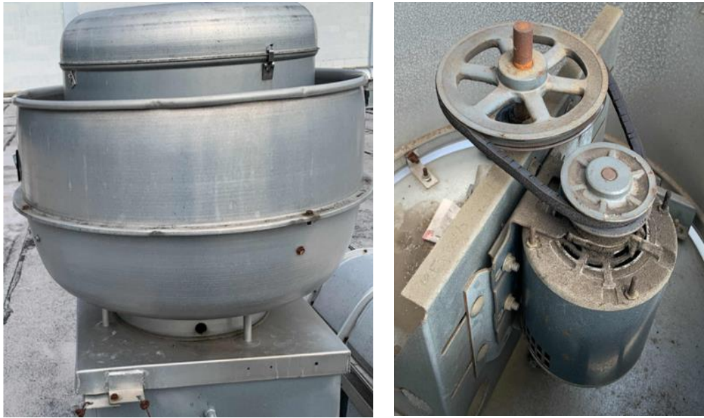
Typical Exhaust Fan
