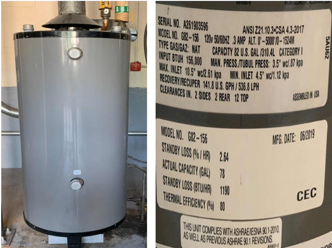
Domestic Storage Tank Water Heater
