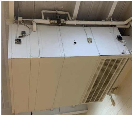
AHU and H&V Unit
