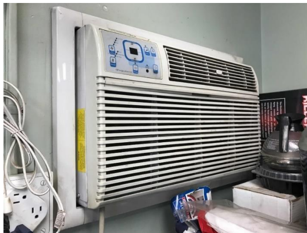
Window AC Unit
