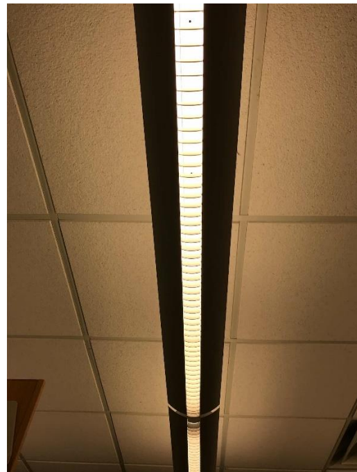
T5 Fluorescent Fixture
