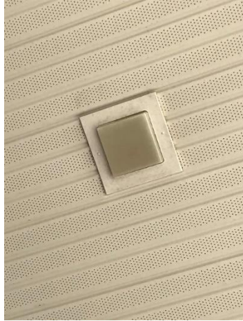
Exterior Canopy Light
