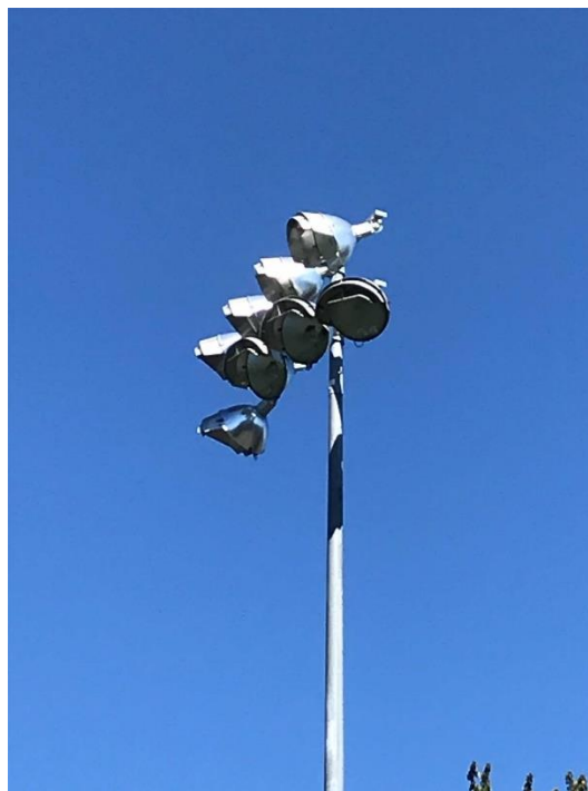
Pole Mounted HID Fixtures
