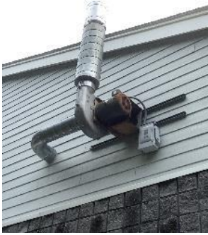
Apparatus Room Truck Exhaust
