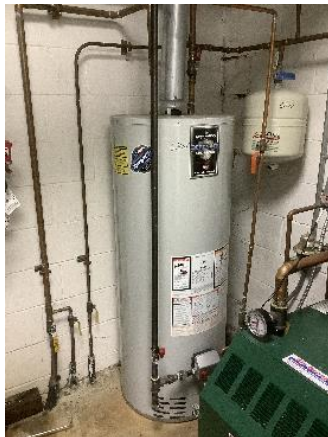
Domestic Hot Water Heater
