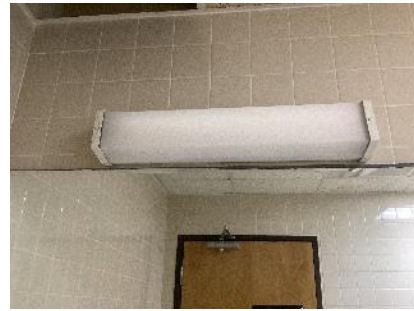
Bathroom Vanity T12 bulbs
