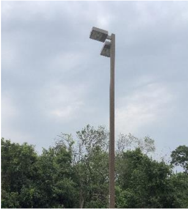
Parking Lot Pole Light
