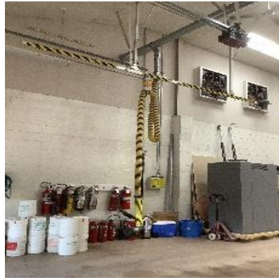
Apparatus Room Fans and Garage Door Motor
