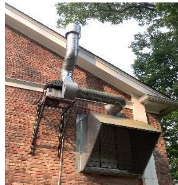
Truck Exhaust Venting System
