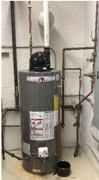
Hot Water Heater
