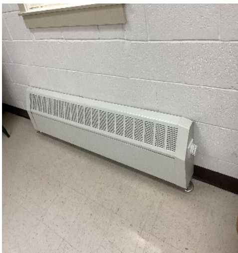
Baseboard Radiator in Kitchen
