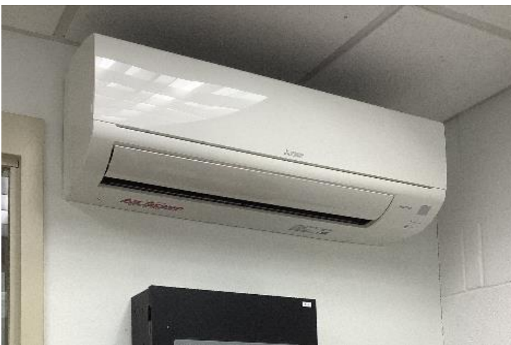
Office Terminal Unit
