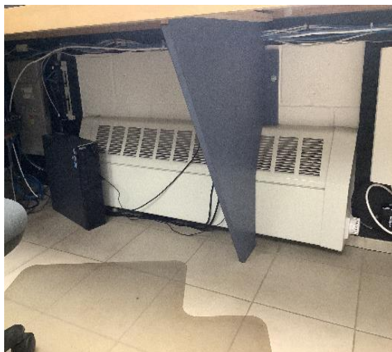
Baseboard Radiator in Office
