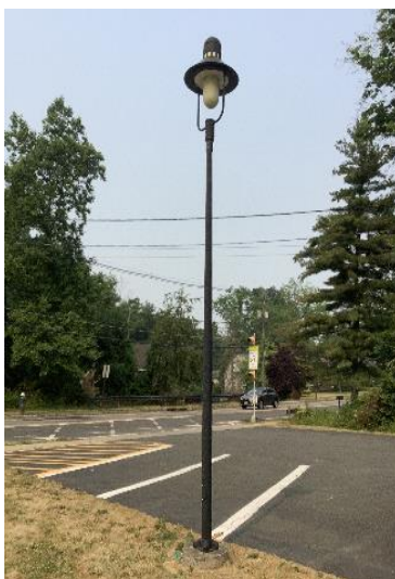
Parking Lot Pole Light
