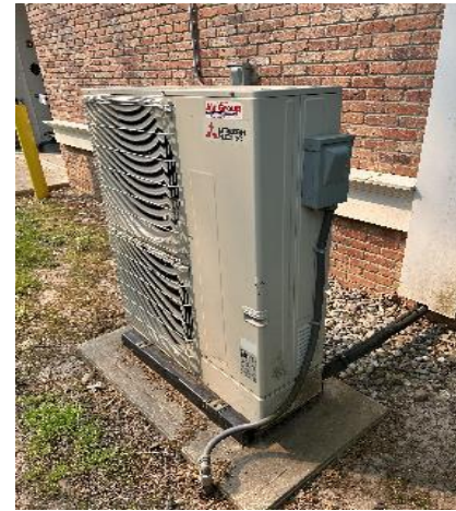
Outdoor Condensing Unit
