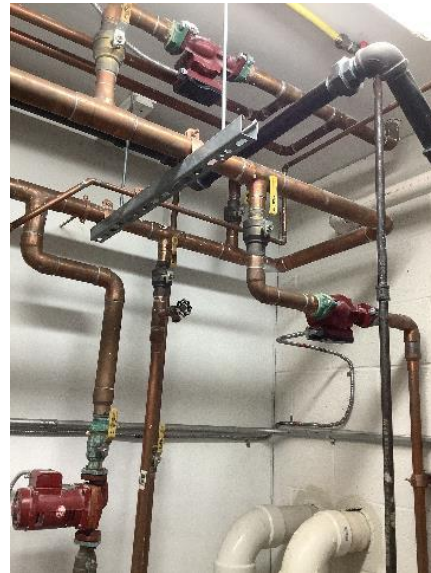
Heating Hot Water Pump and Uninsulated Pipes
