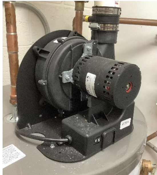
DHW Circulation Pump
