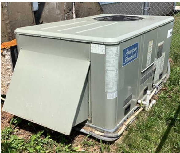
Exterior Ground Package Unit
