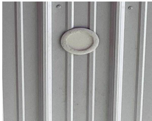
Maintenance Barn – Ceiling Mounted LED Fixture
