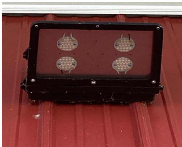
Maintenance Barn – LED Wall Pack
