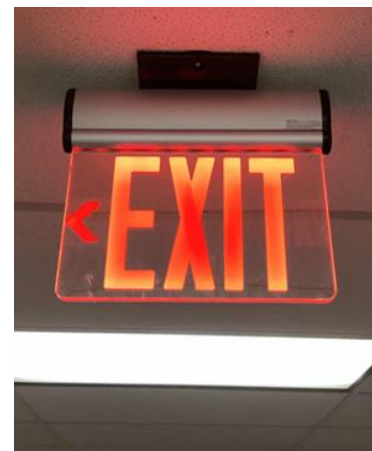
LED Exit Sign
