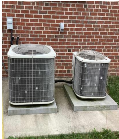
Outdoor Condensing Units
