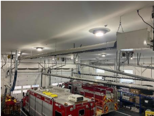
Natural Gas Infrared Heaters in Garage
