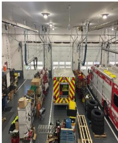
LED Lighting Fixtures in Garage
