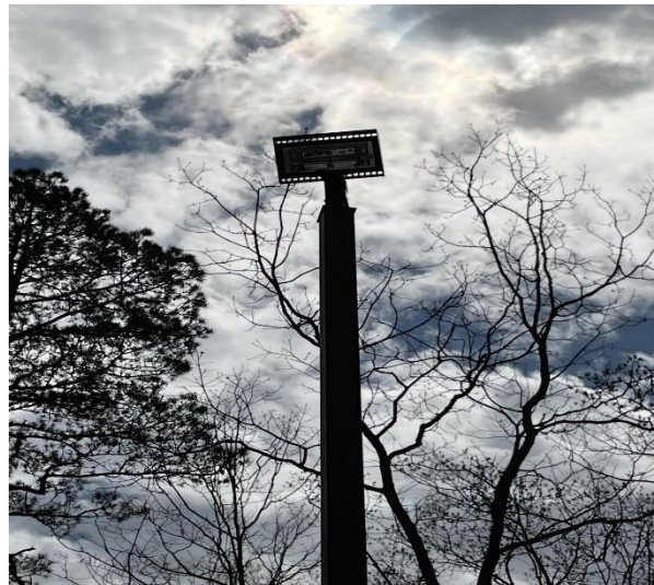
Pole Mounted Parking Lot Lighting
