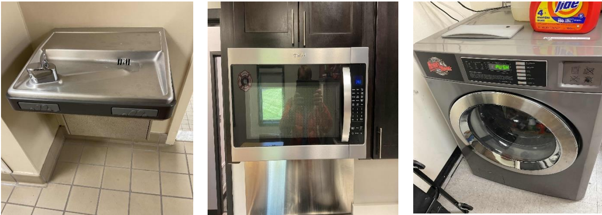
Typical Plug Load Fixtures
