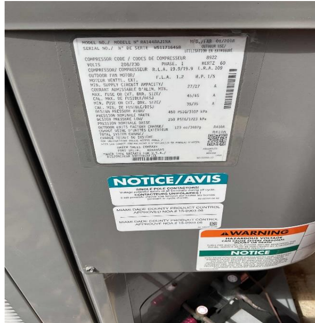
Attached Condensing Unit
