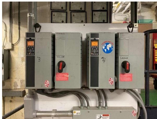
Heating Hot Water Pump VFDs
