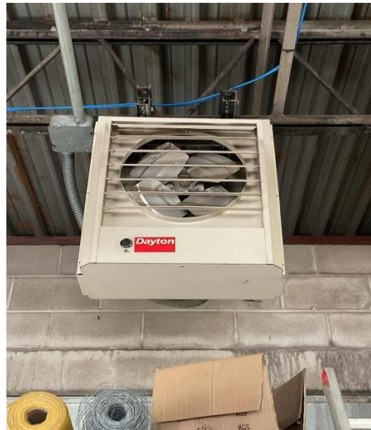
Typical Electric Unit Heater Installed in Garages
