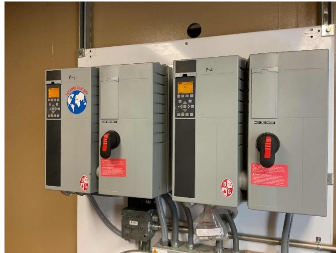
Chilled Water Pump VFDs
