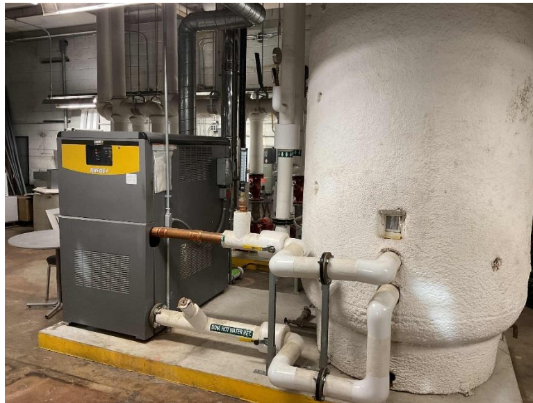
Domestic Hot Water Boiler Configuration & Storage Tank
