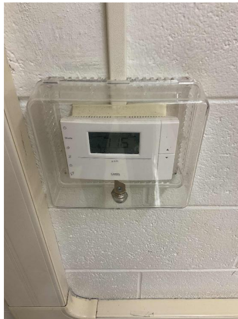
Typical Programmable Thermostat for Local HAVC Control
