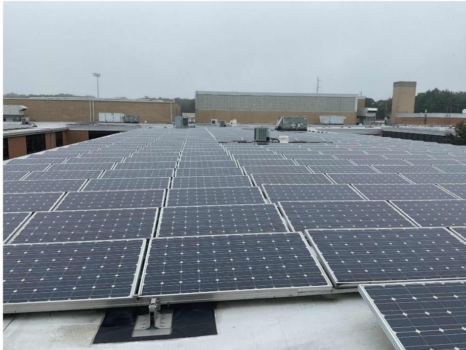
Typical Solar Array Installed on Facility Roof
