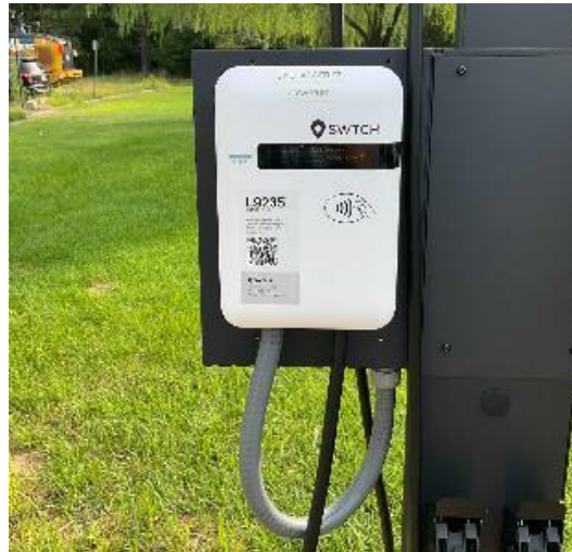
EV Charger – Municipal Building
