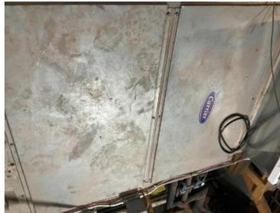
Air Handling Unit
