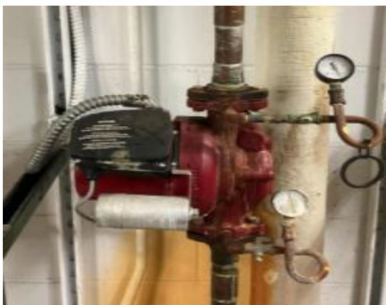
Heating Hot Water Pump
