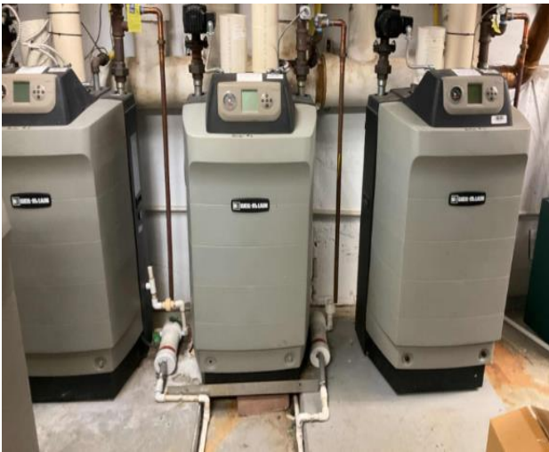
Condensing Modular Hot Water Boilers (Municipal)
