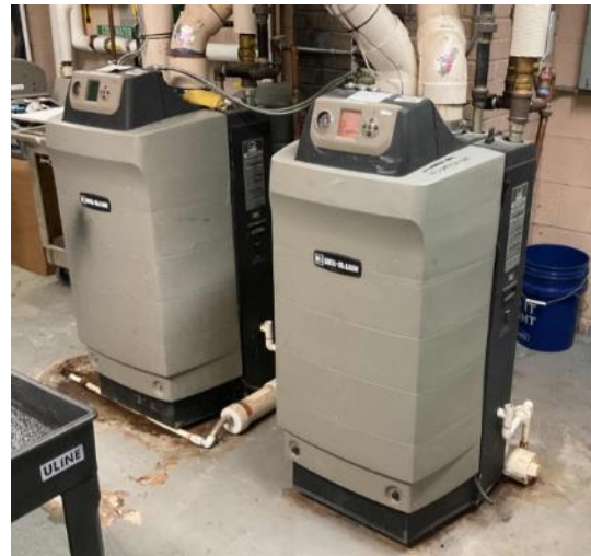
Condensing Modular Hot Water Boilers (Courts)
