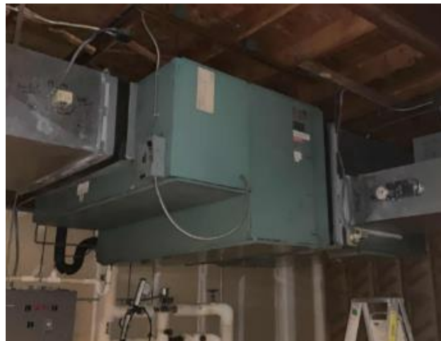
Air Handling Unit
