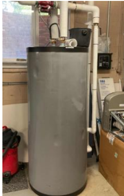
Municipal Building DHW
