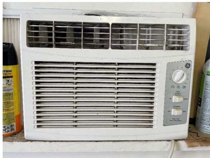
Window AC Unit
