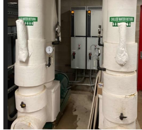
Chilled Water Piping
