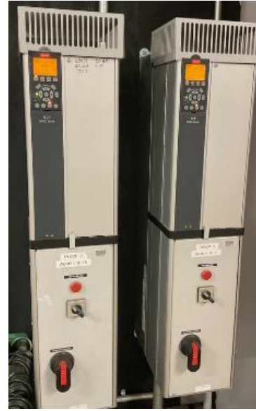
Heating Pump VFDs
