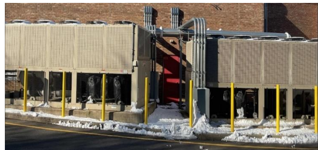
Air Cooled Screw Chillers
