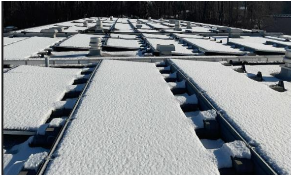
Roof Mounted PV Array
