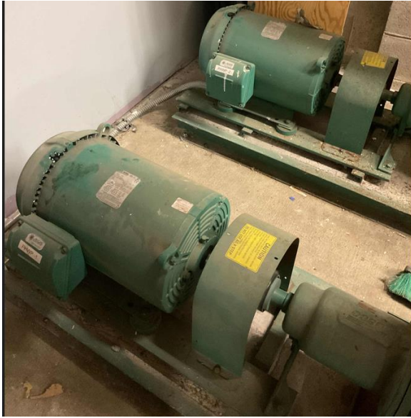
Heating Hot Water Pumps
