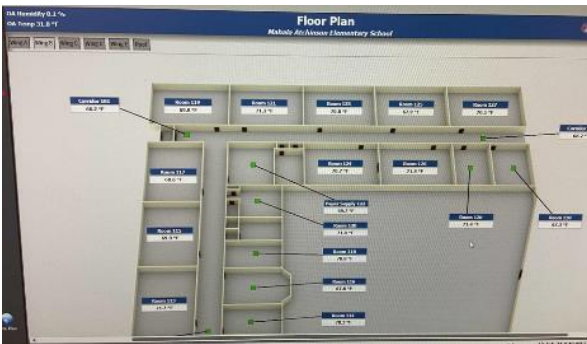
BAS Room Temperature Status
