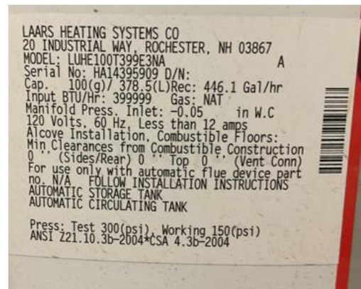
Water Heater Nameplate
