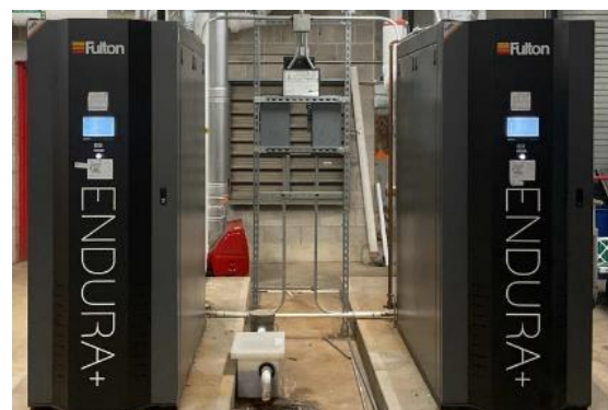
Hot Water Boilers
