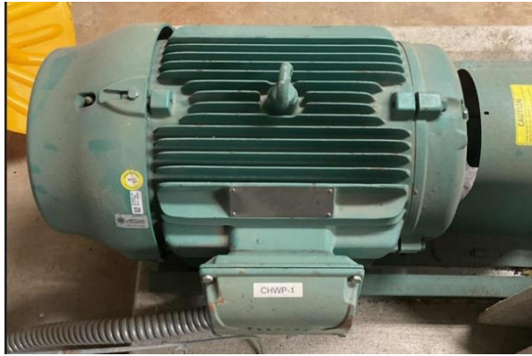
Chilled Water Pump
