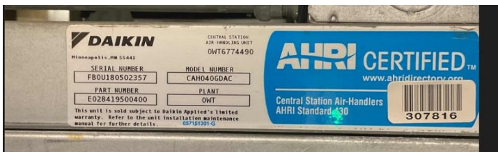
Daikin AHU Nameplate
