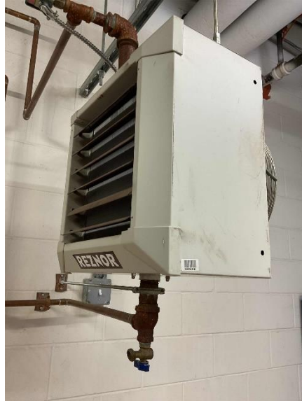
Typical Site Unit Heater
