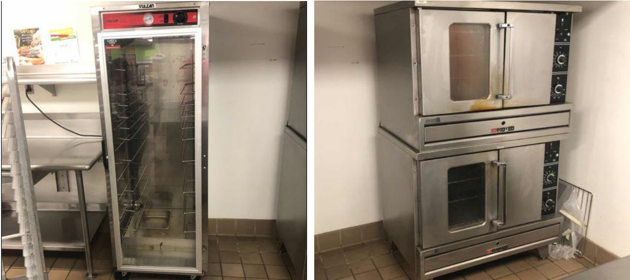
Electric Holding Rack and Oven
