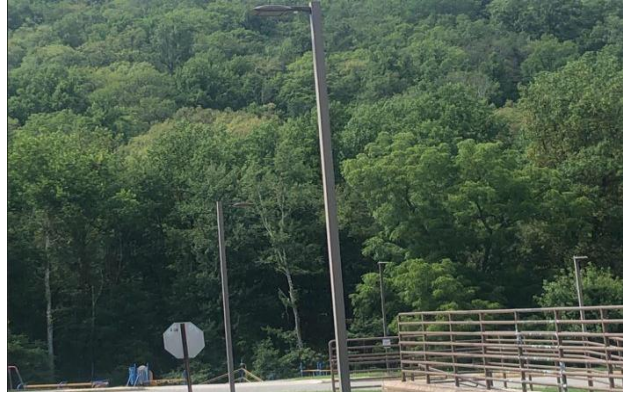
Pole Mounted Light Fixture
