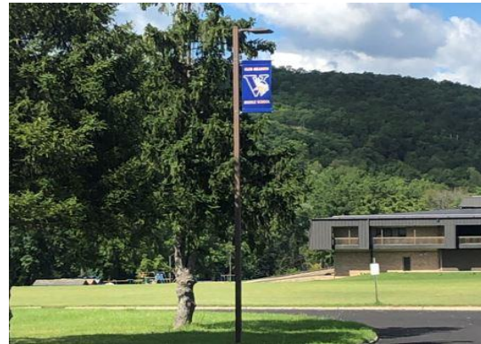
Pole Top Fixtures
