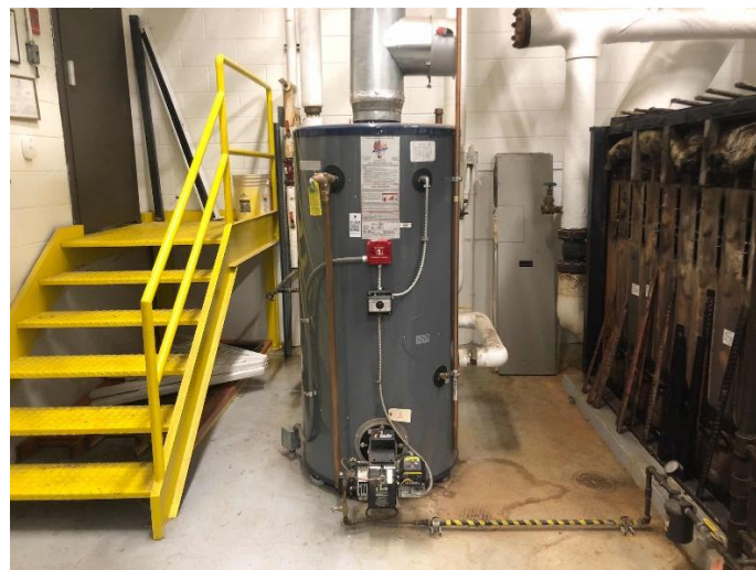
Storage Tank Water Heater
