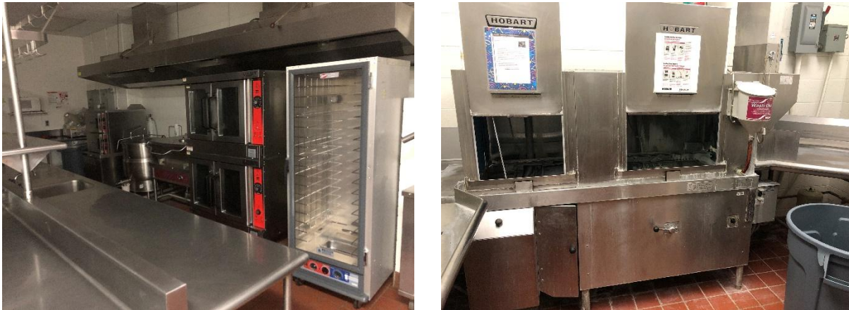
Kitchen Equipment and Dishwasher
