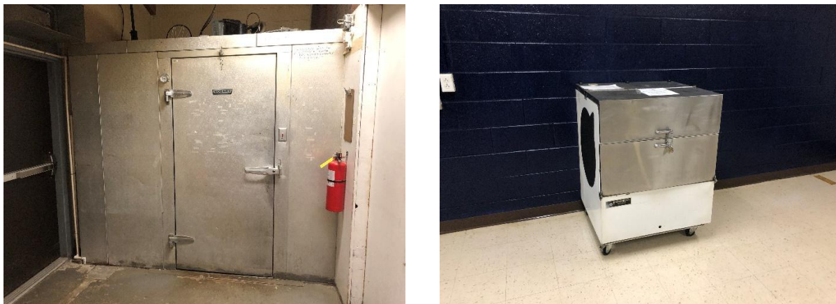
Walk in Cooler and Refrigerator Box
