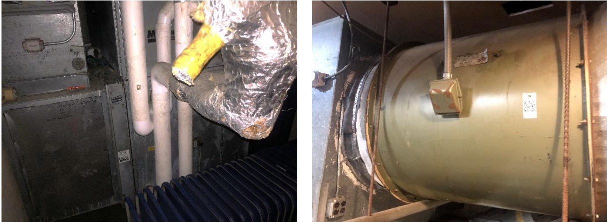
Air Handling Unit
