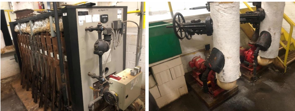
Hot Water Boilers and Heating Hot Water Pumps
