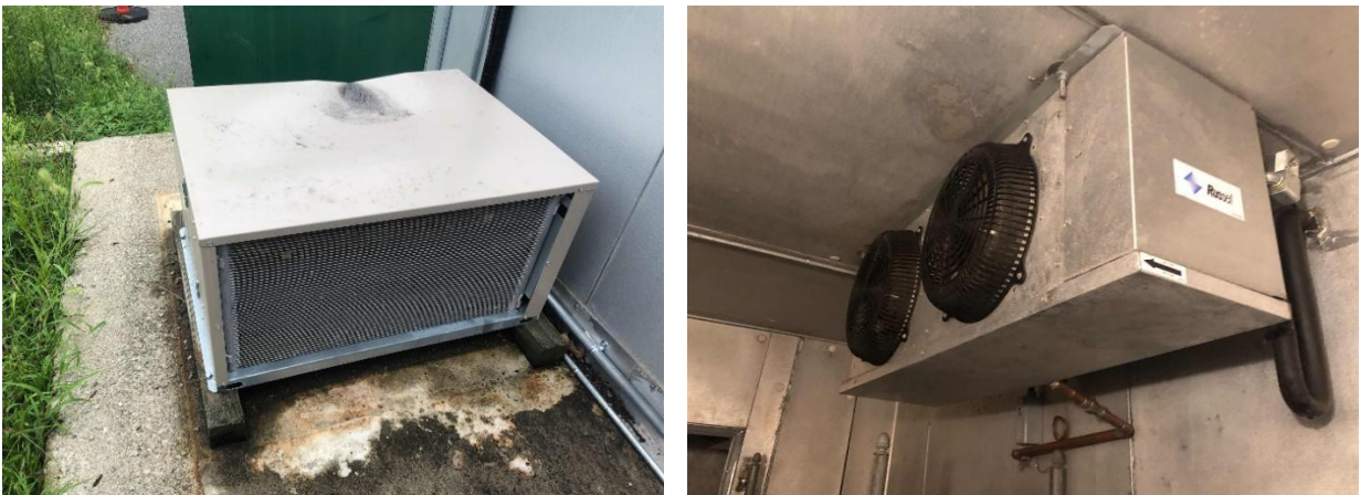
Outside Condensing Unit and Indoor Evaporator Fans
