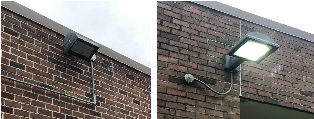
Flood and Arm-Mounted LED Fixtures
