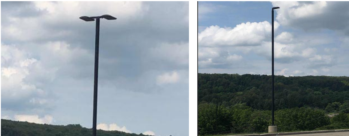
Pole Mounted LED Fixtures
