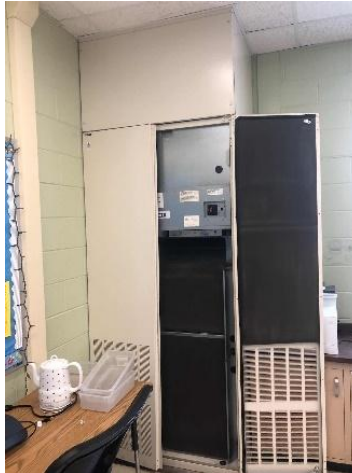
Packaged Air Source Heat Pump
