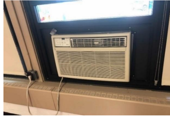
Window AC Units
