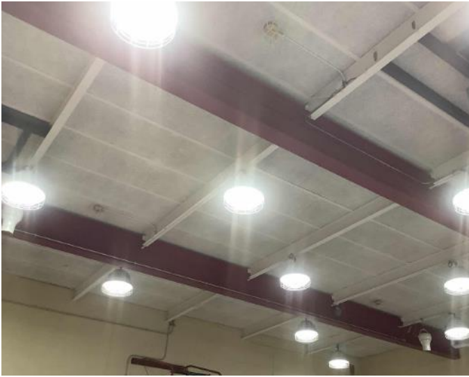
LED Gym fixtures
