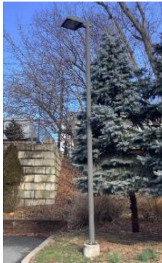
Metal Halide Pole Arm fixture
