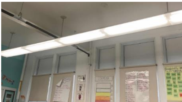
Classroom T8 linear fixtures
