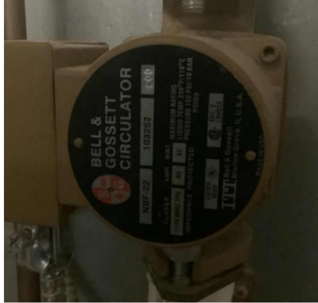
Hot Water circulation pump
