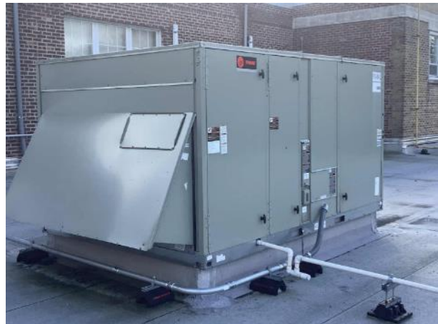
Gym Packaged unit
