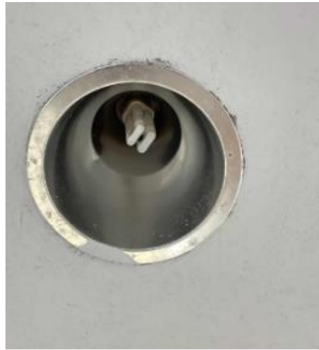
Exterior CFL fixture
