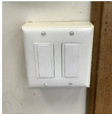
Wall Switch with Remote Occupancy Sensor
