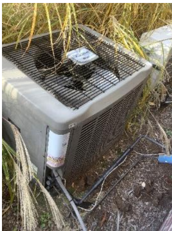
Condensing Unit missing DX Insulation
