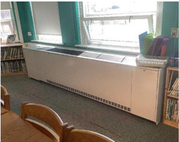
VRF Unit Ventilator - Library
