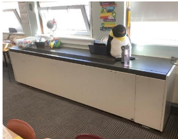
Older Unit Ventilator
