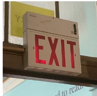
Non-LED Exit Sign
