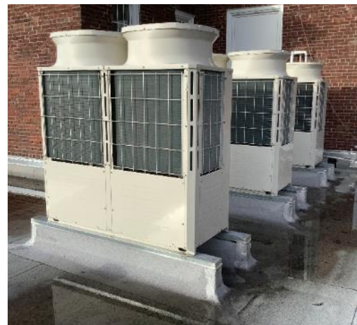
VRF Split Condensing Units
