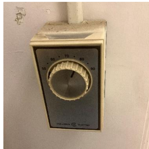
FCU Local Controls
