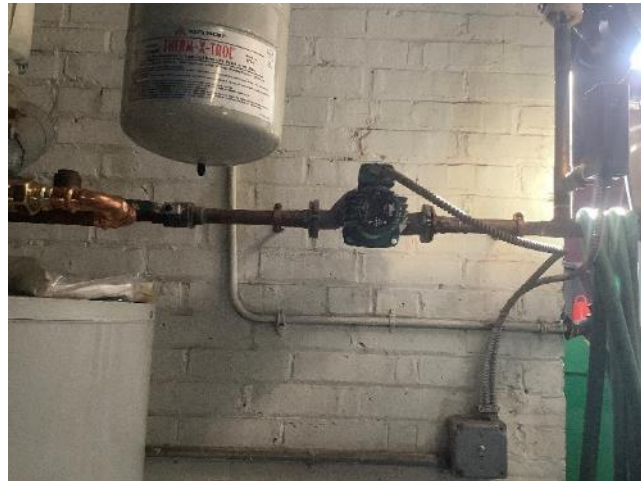
DHW Pump and Uninsulated Pumps
