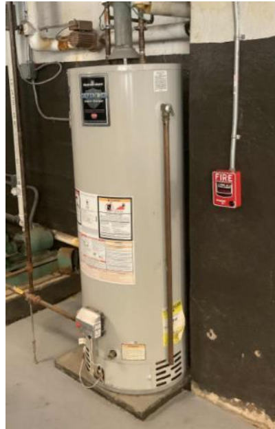
Domestic Hot water heater
