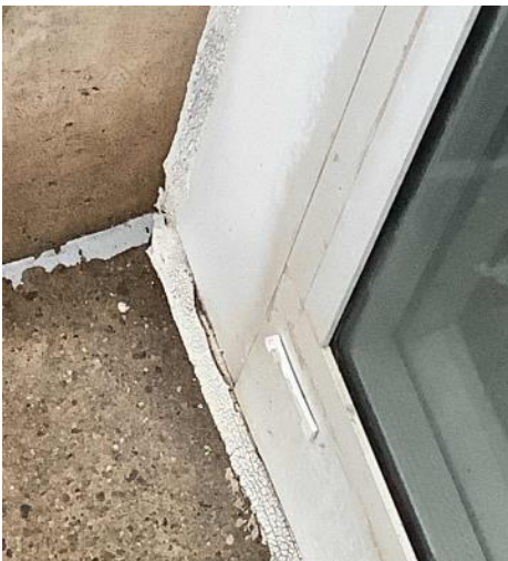
Worn-out window seals
