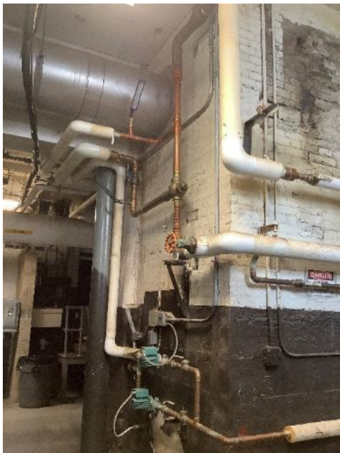
Uninsulated DHW Pipes
