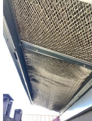
Economizer Grate – RTU-5
