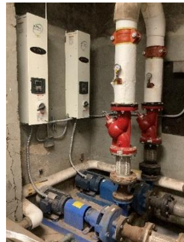
HHW Pump 3 and 4 and VFDs
