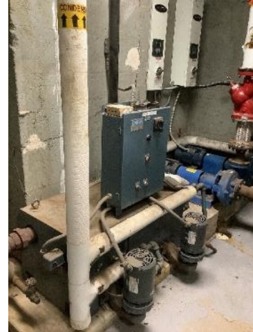
Condensate Return Tank #2
