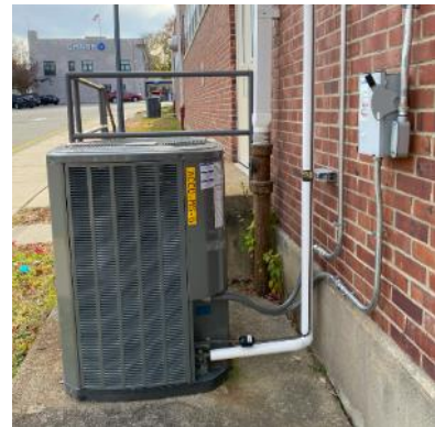
New Condensing Units
