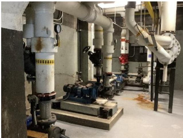
Pumps and Heat Exchanger
