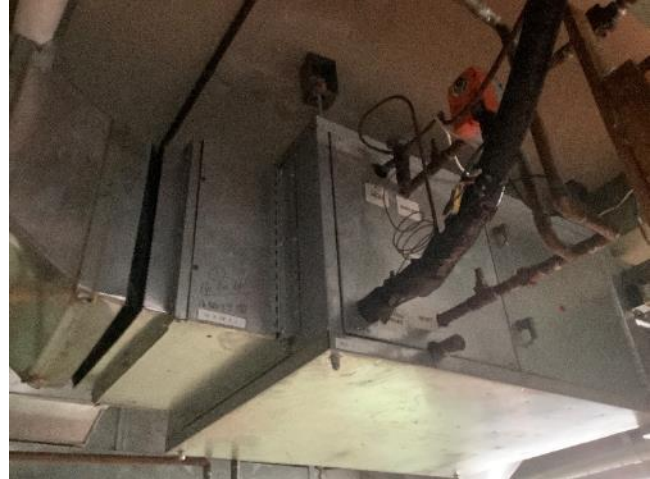
Uninsulated HHW Pipes
