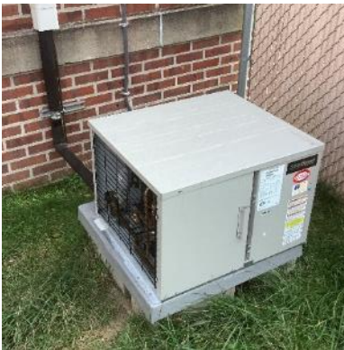
Kitchen Back Rooms Condensing Unit
