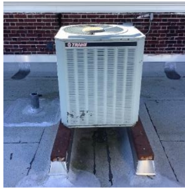
Old Condensing unit
