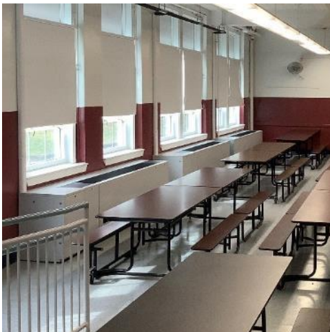
VRF Unit Ventilators – Cafeteria 1
