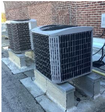
Old Condensing units
