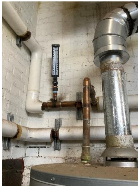
Uninsulated Pipes and Supply Thermometer
