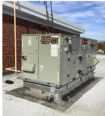
Locker Room RTU
