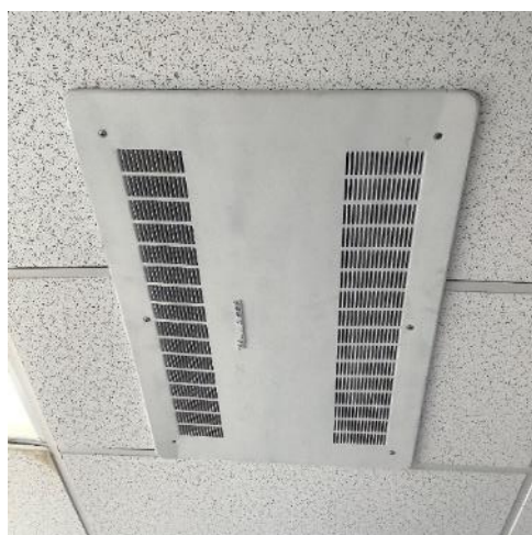
Ceiling FCU - Corridor
