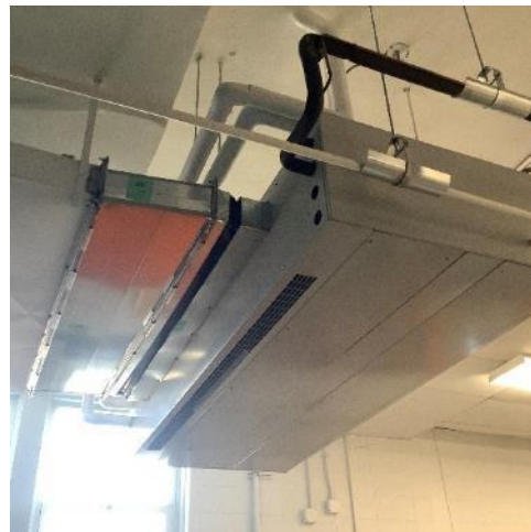
Ceiling Mounted Unit Ventilator
