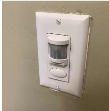
Wall Occupancy Sensor Switch
