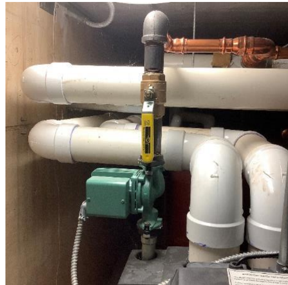
Gym HHW return pump and uninsulated pipes
