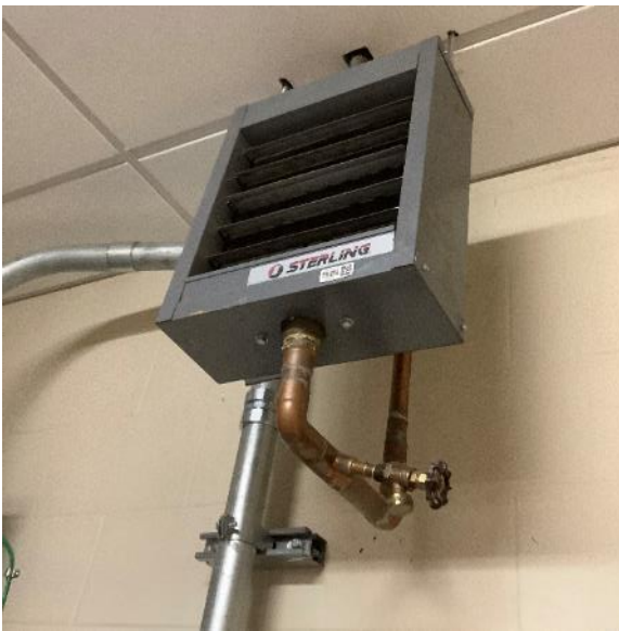
Pendant Unit Heater – Gym Storage
