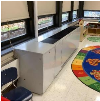
New Unit Ventilators
