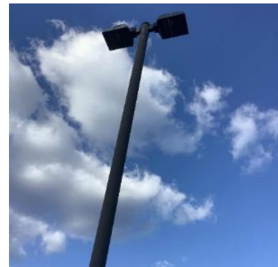
2-Headed Parking Lot Pole Light
