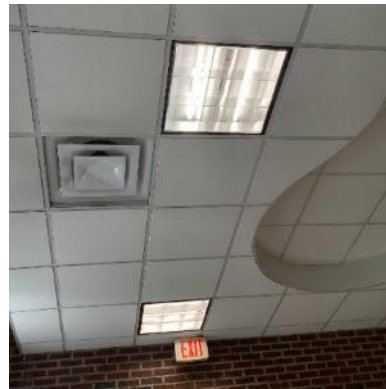
Recessed Parabolic Fixtures
