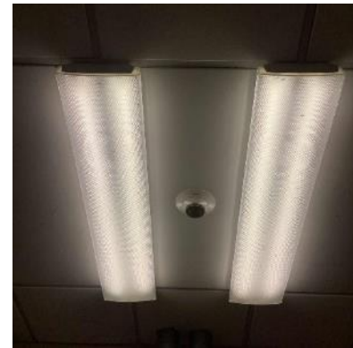
Linear Fluorescent in Gym Storage
