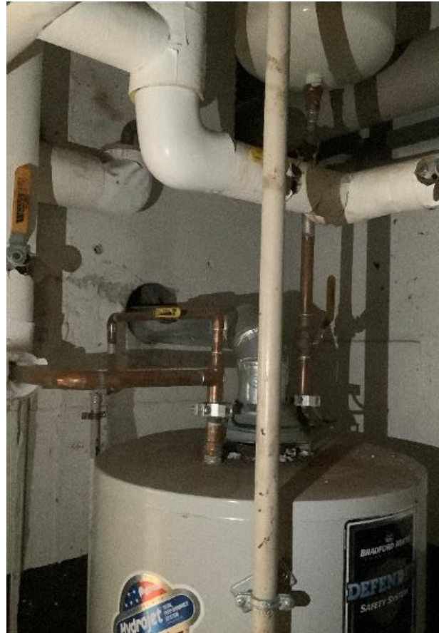
DHW uninsulated pipes
