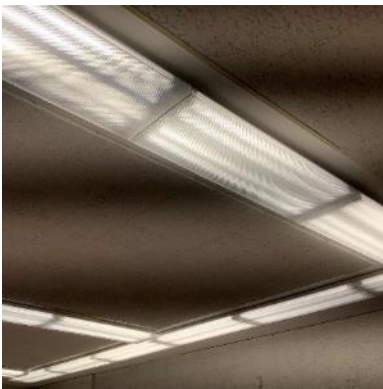
Surface Mounted Wrap with LED T8 Tubes
