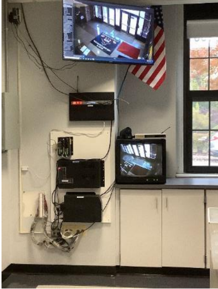
Security Equipment – Main Office
