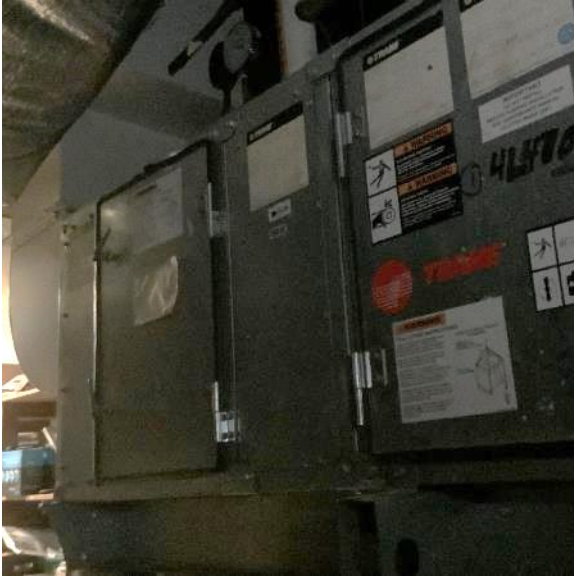
Multipurpose Room AHU
