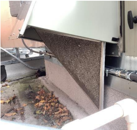
Economizer on RTU-LN-2
