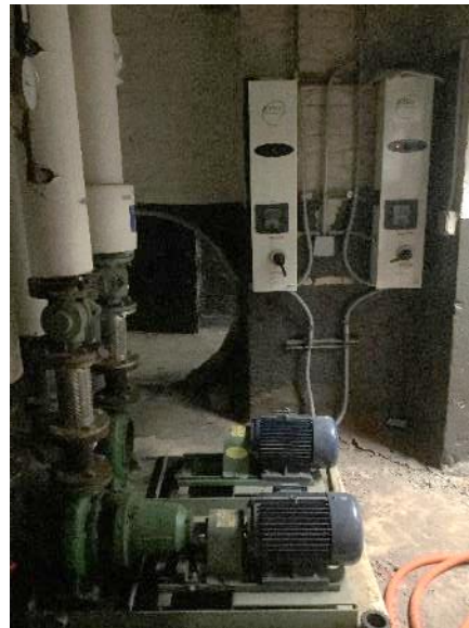
HHW Pump 1 and 4 - VFDs
