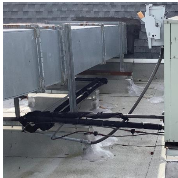
AC-1 DX lines – poor condition
