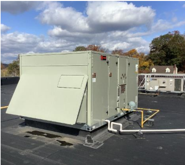
RTU-LN-1 and RTU-3
