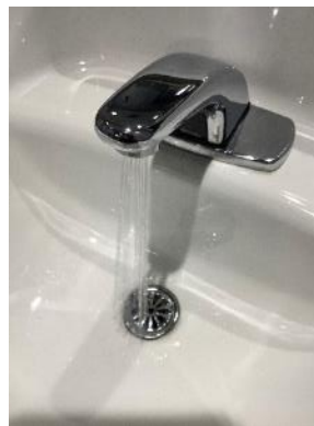
Low Flow Restroom Sink
