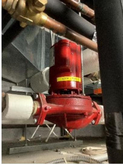
HHW Pump Loop 1
