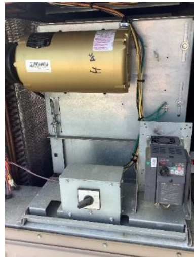
Supply Fan Motor with VFD
