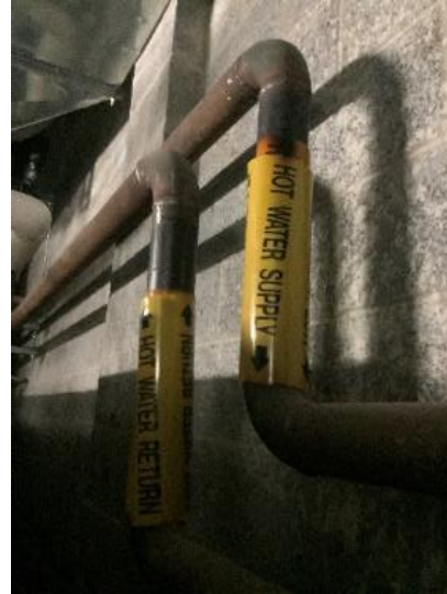
Uninsulated HHW pipe – Fan Room #2
