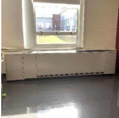
VRF Unit Ventilator
