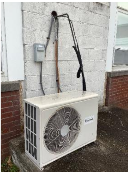
Mini-Split with Missing DX Insulation
