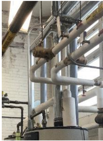
DHW Circulation Pumps
