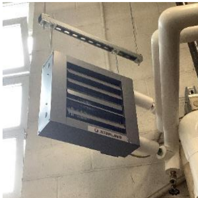
Boiler Room unit heater
