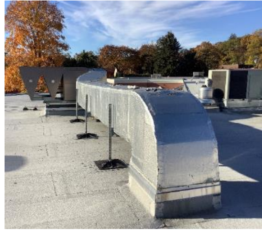
RTU and RTU-4
