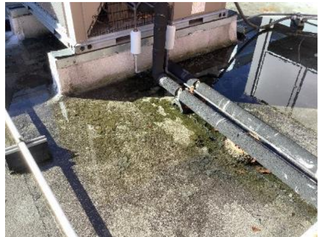
Water and Moss Buildup on Roof
