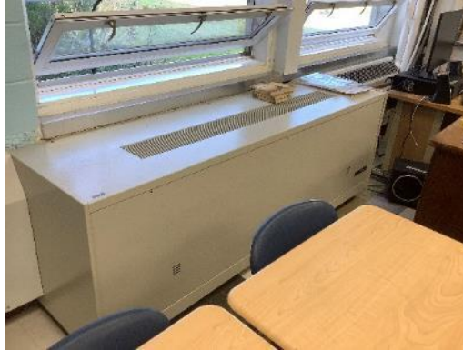
Old Unit Ventilator
