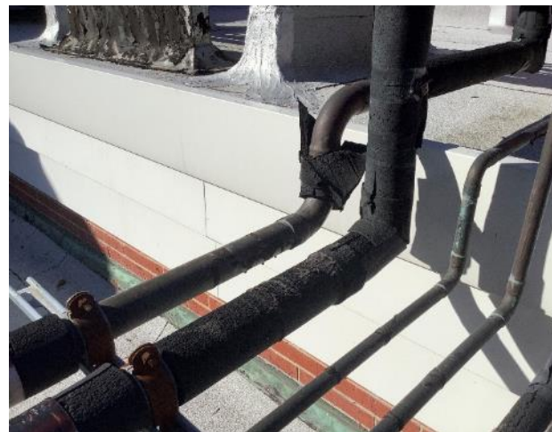
ACC-1 Missing DX Insulation
