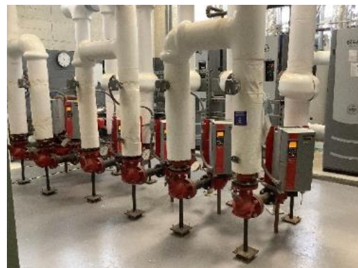
HHW Pumps and VFDs
