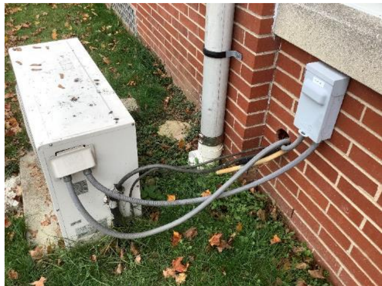
Mini-Split with Missing DX Insulation
