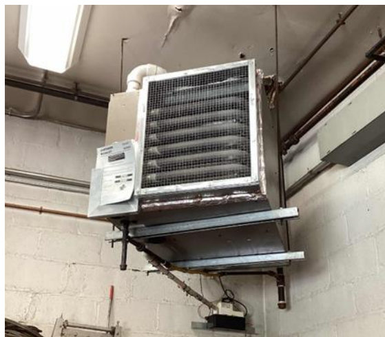
Garage Forced Air Furnace
