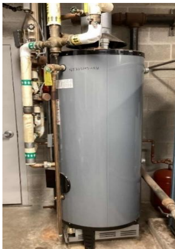
Main Building DHW Heater
