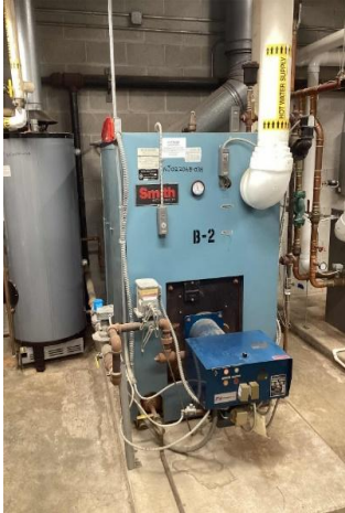
Non-condensing Hot Water Boiler
