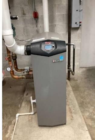
Condensing Hot Water Boiler
