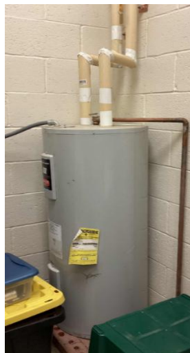
Annex DHW Heater
