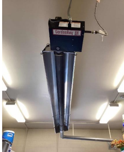
Annex Garage Infrared Heater
